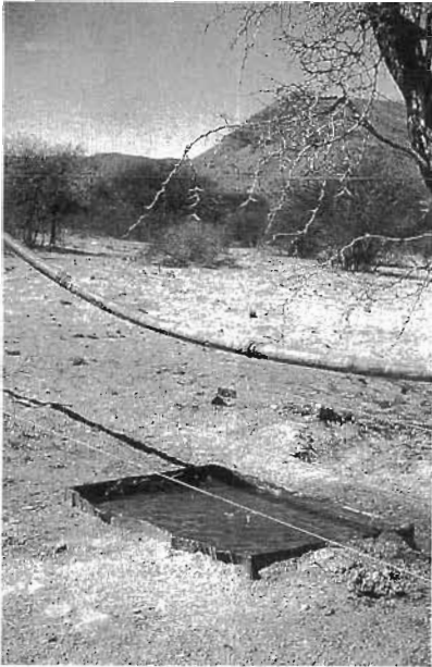
Photo 23-3 Water pipeline strung along a fence to avoid damage by porcupines. A leak has developed and been turned to advantage as a watering point for birds and small animal life. Namibia (courtesy Argo Rust).
