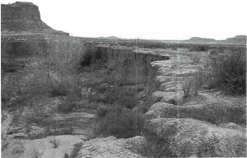
Photo 20-6 Fifty years of total rest in a very brittle, low-rainfall environment. Most grass is already dead, bare ground and soil erosion are extensive, and many shrubs are dying. The main plants left are algae and lichens. Chaco Canyon National Park, New Mexico.
