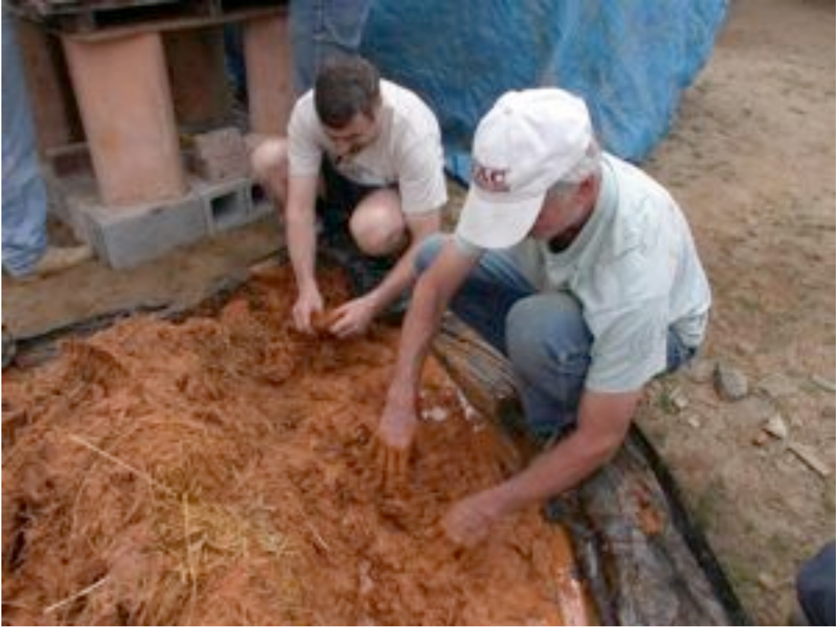
John and Tom prepare cob. Water is added and the mix is worked into bread loaf shaped lumps that are laid on the form
