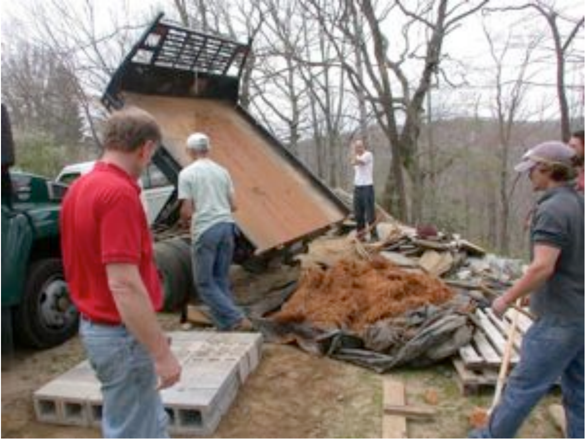
Tom Trout has brought a load of local clay from an excavation site mixed with straw.
