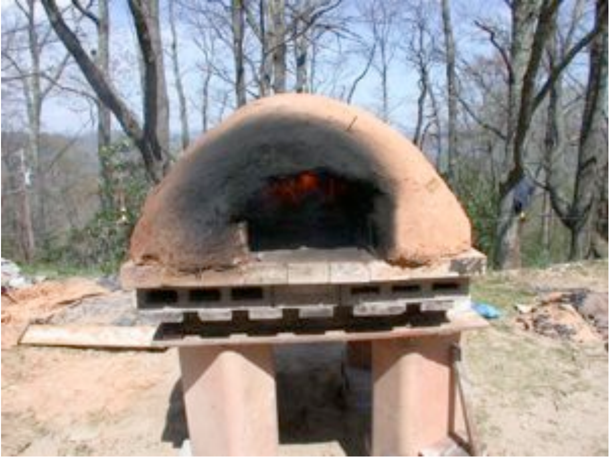
Sand is gone, and the front of the oven is dry.
