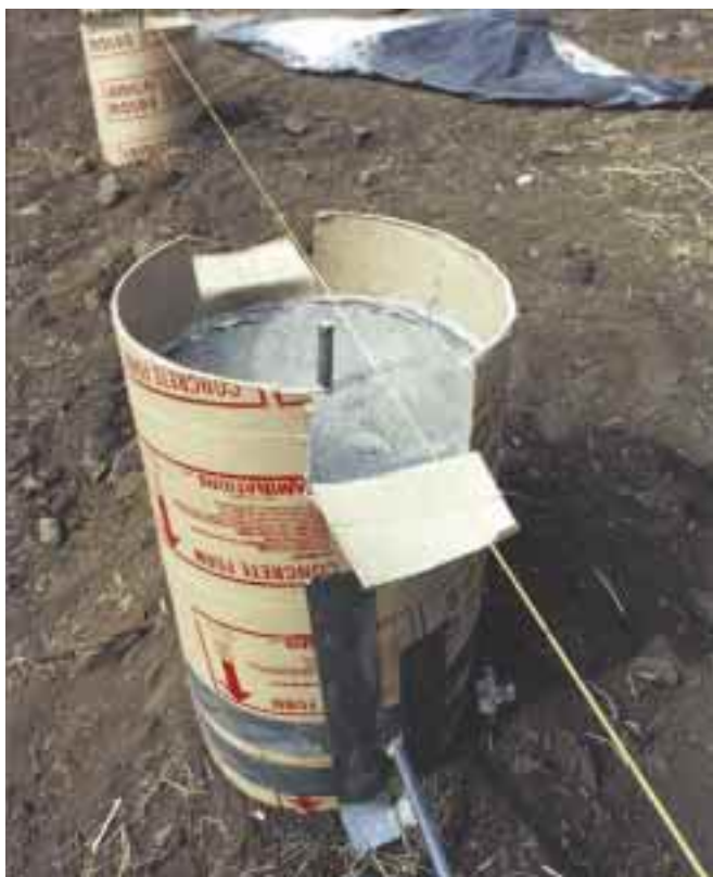
Above: Twelve inch concrete piers extend below frost line. Rebar prevents lateral movement of posts.
