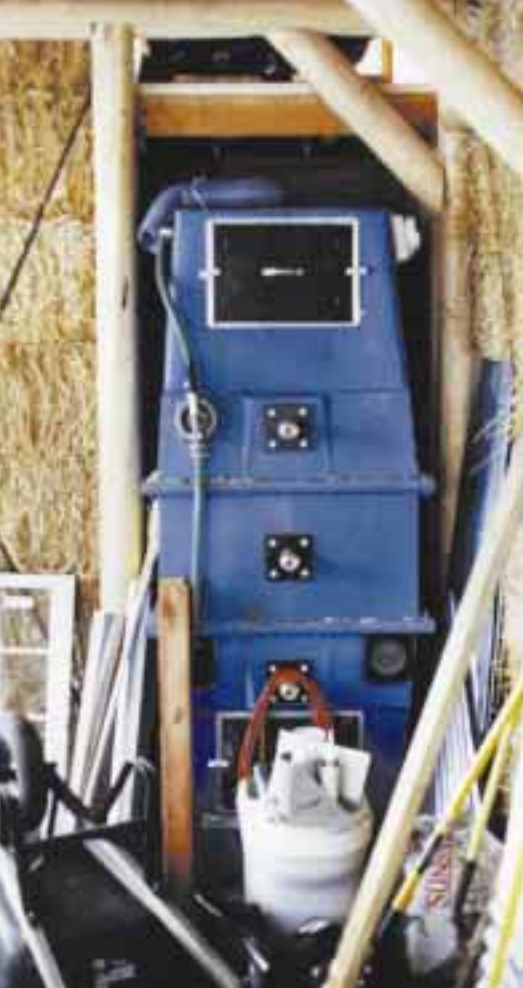
Above: Big Blue, the composting toilet, in the bottom of the Tower of Turd (surrounded by the usual construction clutter.) Vents above the tank allow warm air into the second floor, taking the chill out of winter duties.
