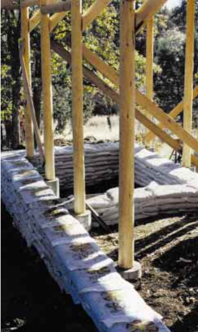
Above: Dirt bag retaining wall/footing along north wall and under future bathing deck.
