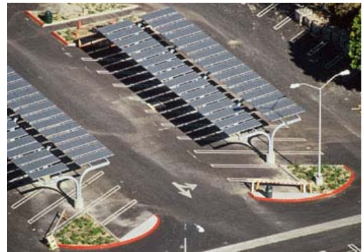
Commercial solar-covered parking lot example
