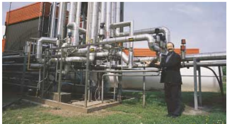
RMI's Amory Lovins showing typical inefficient pipe layout while consulting with HP Bulmer, Ltd., England. Photo: Cameron M. Burns
