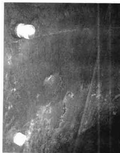
Giant sheets of rust peeling off the inside of an old galvanized bolted steel tank. Upper inlet has brass nipple in it; the lower inlet has a PVC male adapter. In each case the function is to keep the threads usable.
