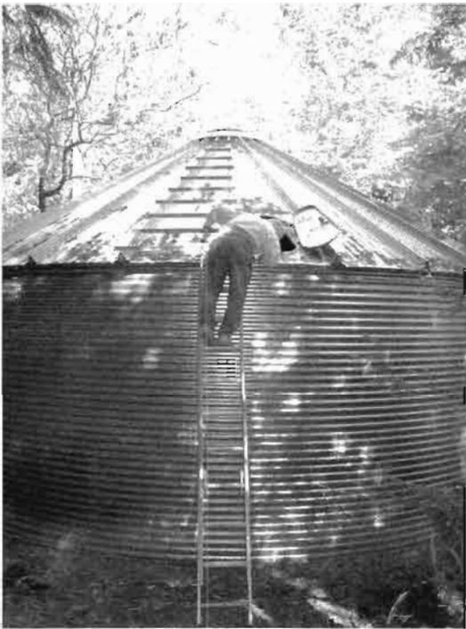
The access on this 50,000 gal (190 m 3 ) galvanized/poly bag tank is from the top only, as a perforation of this size of the liner would not be a good idea. Attempting to fill the 8,000 gal (30 m 3 ) or so of space under the lightweight conical roof with water would be equally inadvisable.
