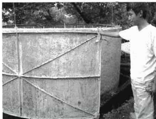
Pulling reusable steel forms off of a new concrete tank in a Mexican village.
