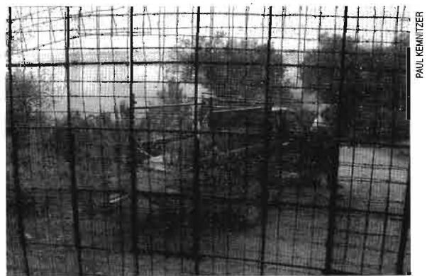
Close-up of wall armature; 1/2" rebar on 1' centers, two layers of 6" x 6" mesh, offset to make 3" squares, sandwiched between expanded metal lath on one side and chicken wire on the other.
