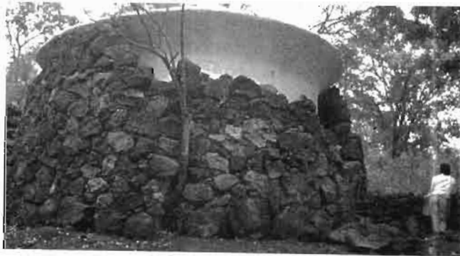
Aesthetic shield of rock around a 13,000 gal (50 m 3 ) ferrocement cistern.
