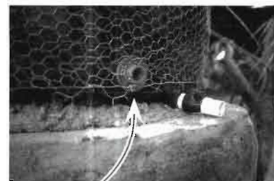
250 gal (1 m 3 ) HDPE drinking water tank with new bulkhead fitting outlet and chicken wire ready for stucco. (See also Plastic Tank Drain Retrofit, p. 60.)
