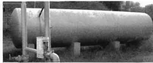
A huge pressure tank for a water system that serves about
