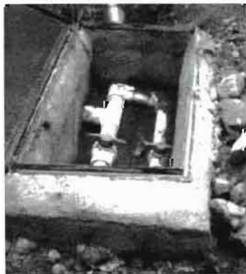
Valve box with locking metal lid, made of brick in Mexico.
