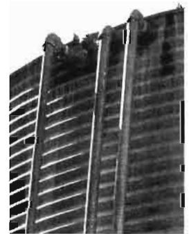
Separate inlets from two wells, and an overflow all the way at the top of a riveted, corrugated galvanized tank.
