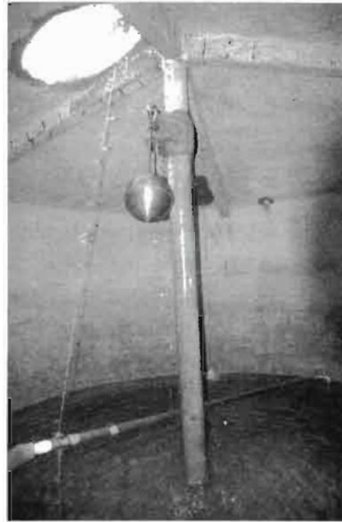
Same tank inside. A ladder could have been incorporated in the central pillar, for safety and to avoid the hassle of feeding an extension ladder into the tank.
