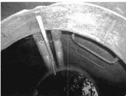
Ladder made of 1/2", epoxy-coated, grade-60 rebar integrated in a ferro-cement water tank. This choice of rebar reduces the two main problems with rebar ladders: bent steps (grade 60 is half again as strong as standard grade-40 rebar) and rusting away, which can render the ladder unsafe as well as impact the structural integrity of the tank wall.
