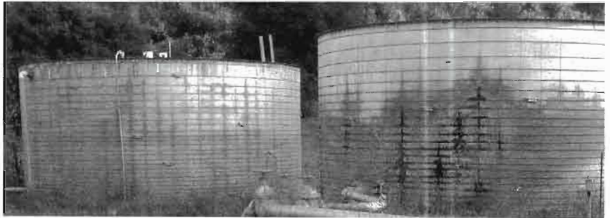
Two 70 year old redwood tanks, one leaking, one not. The water in this system is highly sulfurous and quickly corrodes galvanized tanks.
