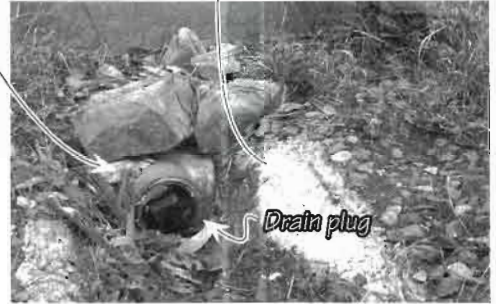
The completed drain was stoppered with a 4" plug (a cap would be better.) The concrete around the drain takes the pipe wrench torque from removing the plug, so the drain doesn't twist and tear out of the bottom of the tank.
