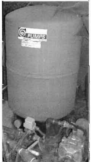
Pressure tank and pressure pump.
