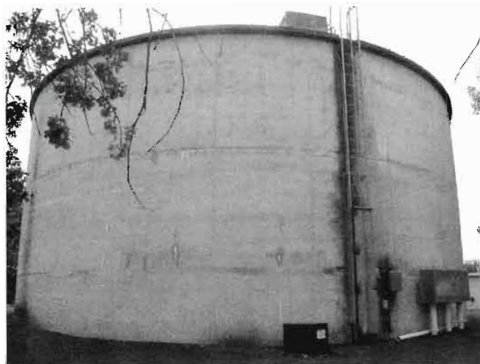
Large concrete water tank at a retirement community of 2,000 members in Oregon.
