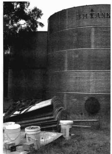
A good quality, 50+ year old bolted steel galvanized tank (with smooth surface, in background) and a less than 15 year old cheap, riveted galvanized steel tank (with corrugations, in foreground). Though much newer, the cheaper tank shows signs that it will fail before the older, higher quality tank. The pile of parts in the foreground is for another good quality, bolted galvanized steel tank.
