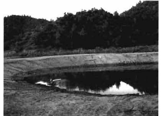
Construction of a 100' (30 m) diameter embankment pond in the Cuyama Valley, California. It is filled by gravity with water from a creek diversion, through a mile of 2" pipe. It is used for swimming and emergency storage.
