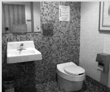
The instructions above the composting toilets tell the user to add some wood shavings after each use.
