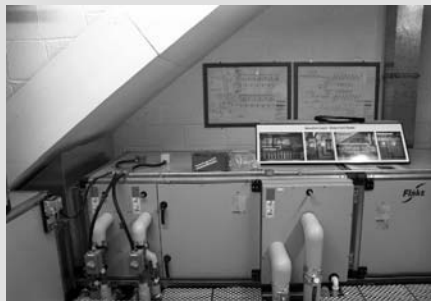
As part of BCZEB's educational remit, the plant rooms display information panels explaining the operation of the building systems.
