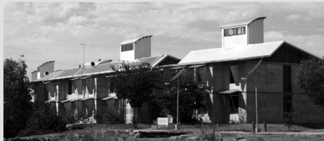
The central vents, clearly visible over the roofs of the naturally ventilated teaching block, are used to draw air from the air inlets under the windows.
