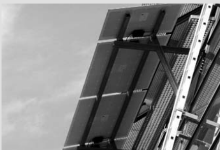
PV panels on steel supports shade the glazed façade.
