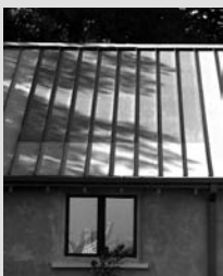
The amorphous PV cells are made of plastic rolls attached to the metal roof substrate between the metal upstands.
