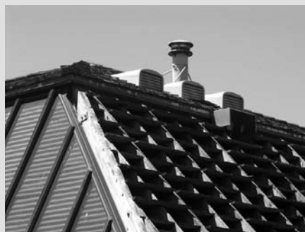
The six air vents and the flue from the wood-burning stove are located on the roof.
