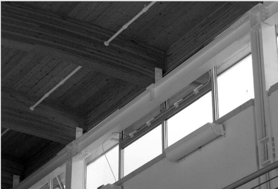
Automatic high level vents.
