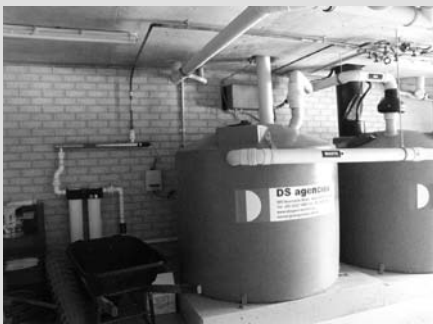
The tanks can be seen in the basement where there are also panels with information on the hybrid toilet system.
