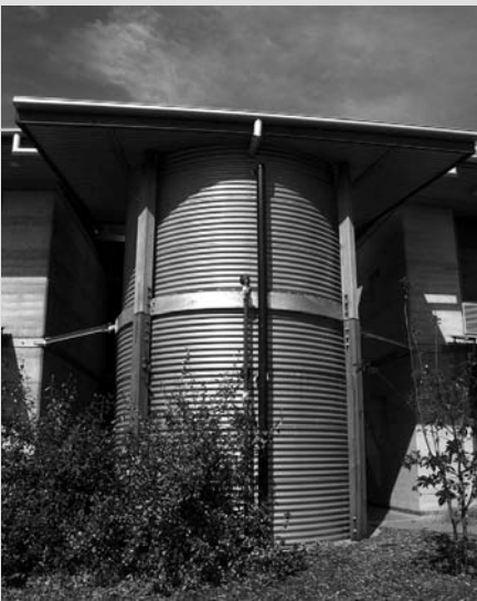
The double-storey rainwater collection tanks have to be strapped back to the building structure.
