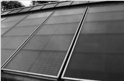
The BCZEB 54m 2 thermal PV array produces both hot water and electricity. The efficiency of conventional PV panels drops as their temperature rises. The thermal PV panels used at the BCZEB have a copper heat exchanger filled with water and glued to the back of the panel and painted black. The heat absorbed by the panel can raise the water temperature to about 25°C, and removing the heat from the PV panel ensures the PV-generating efficiencies remain constant.
