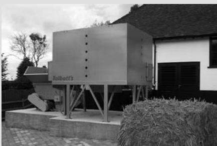
Biofuel is used to heat the building
