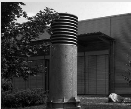
The air intakes, which draw air into the underground ducts are located outside the manufacturing building.
