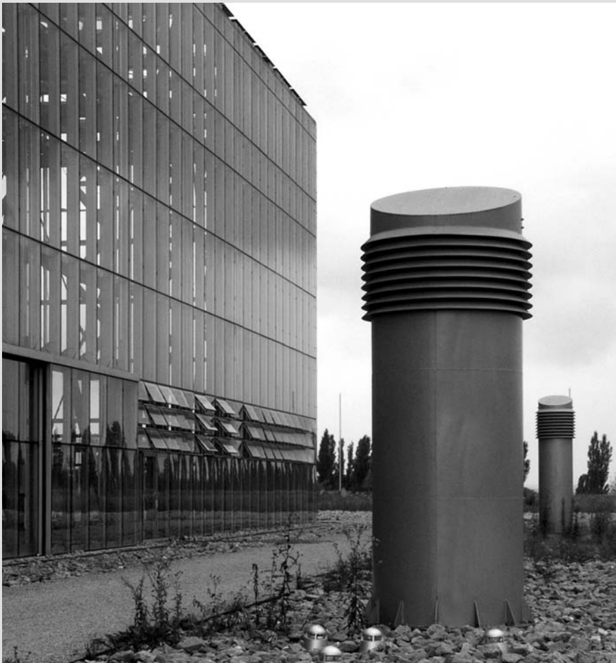
Earth ducts, used to supply fresh air into buildings, take advantage of the earth's constant temperature to heat the incoming air in winter and cool it in summer. The intake ducts here are at the Akademie Mont-Cenis (see p.243).
