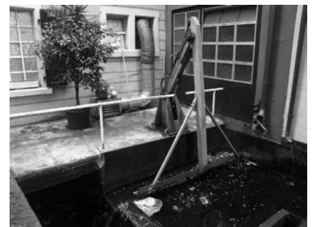
In the centre of Freiburg, two micro-hydro installations, one installed in 1927, the other in 1948, both refurbished in 1992, provide a total of 25,000 kWh/yr and save 15 tonnes of CO 2 emissions.
