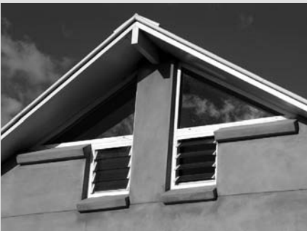
Louvred openings on the west façade allow the cool sea breeze into the building and the hot air out of the building.
