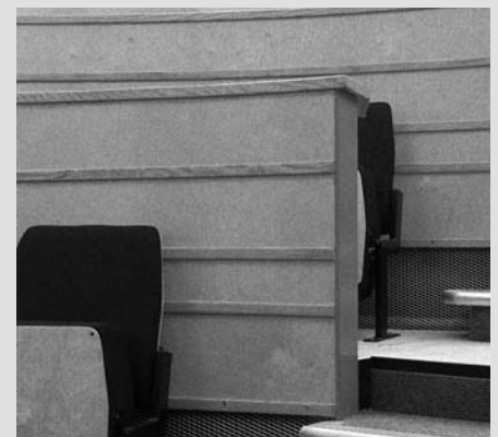
The air grilles are located below the timber panels behind the chairs.
