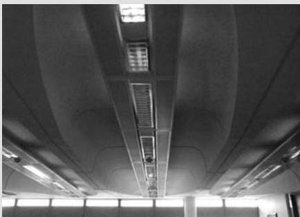
The exposed ceiling coffers house the lighting rafts and smoke detectors.
