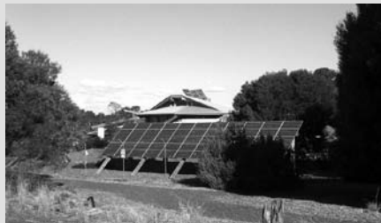
View of the ground-installed photovoltaic array with the Environment Centre behind.
