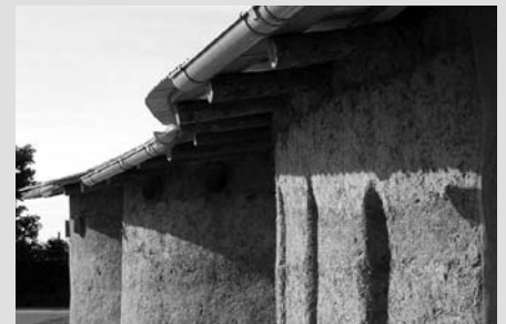
Rainwater is collected in a standard rainwater gutter.
