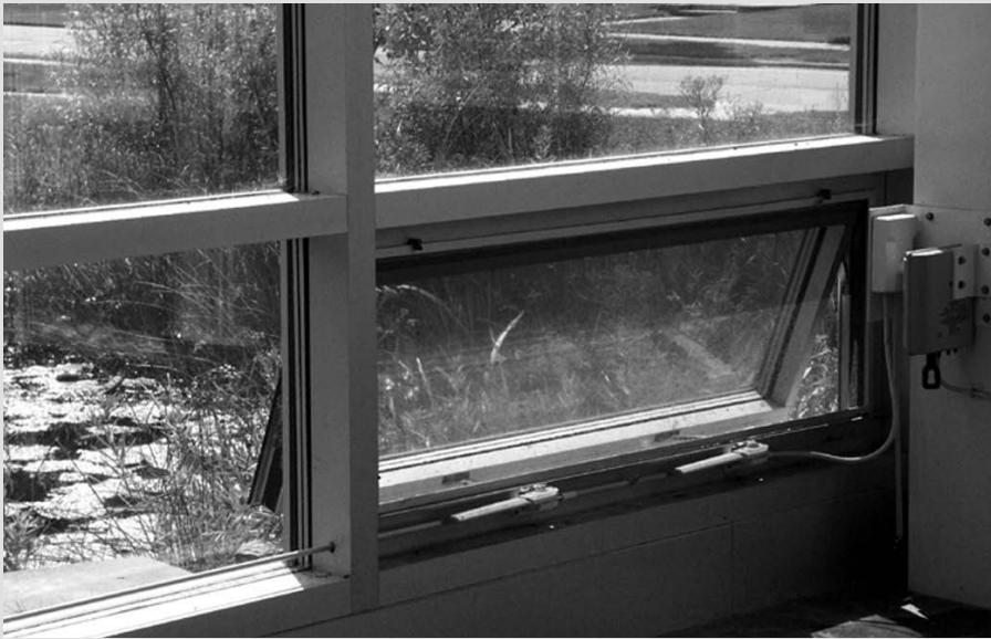
Low level vents with actuators.
