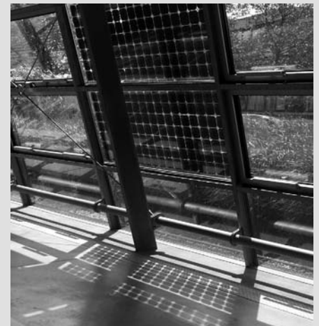
Two building-integrated PV panels between two opening vents.
