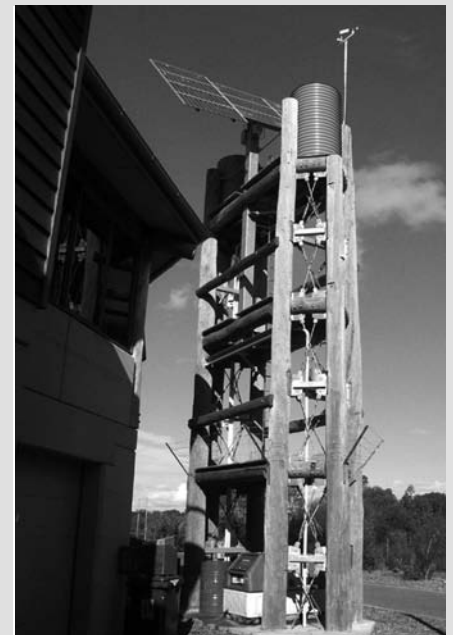
A tower houses the vegetable oil generator and a PV which tracks the sun throughout the day to maximise exposure.
