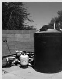
The greywater tank is located outside the utility room.
