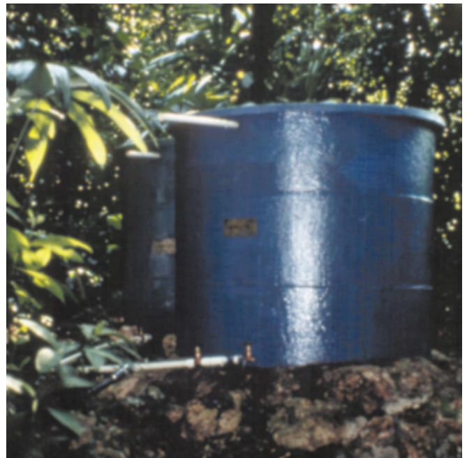
Above: Two 600 gallon water tanks sit 60 feet above the clinic and provide gravity pressure.
