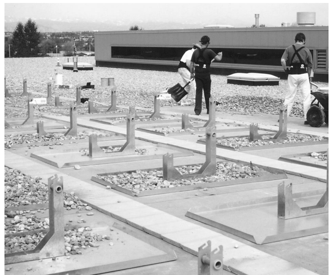
Above: Gravel holds roof jacks to roof.
