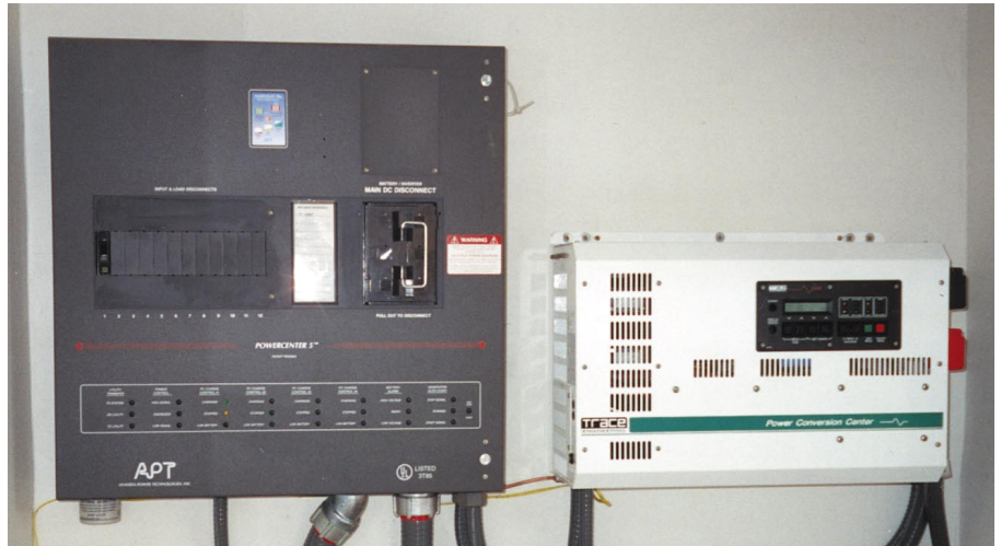
Above: The Ananda Powercenter 5 and the Trace SW4024 are mounted in a separate room from the batteries.
