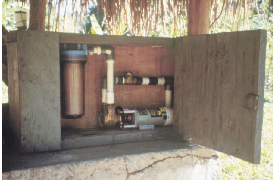
Above: Pump box containing Slowpump™, in-line filter, and Linear Current Booster™ supplies water from a spring. See the pump house on the cover.
