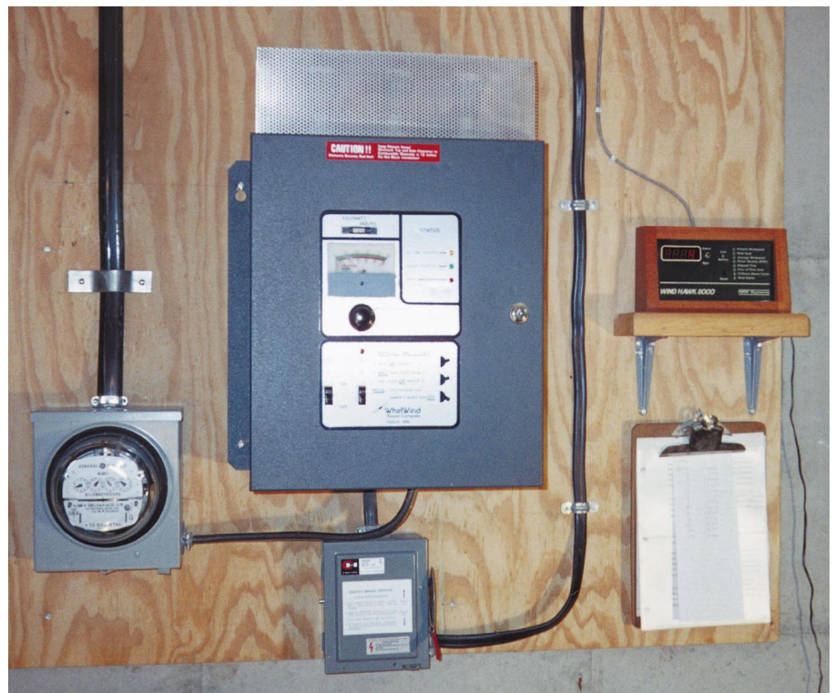
Above: Output Meter, synchronous inverter, safety brake switch, and Wind Hawk 8000 are located inside the house.
