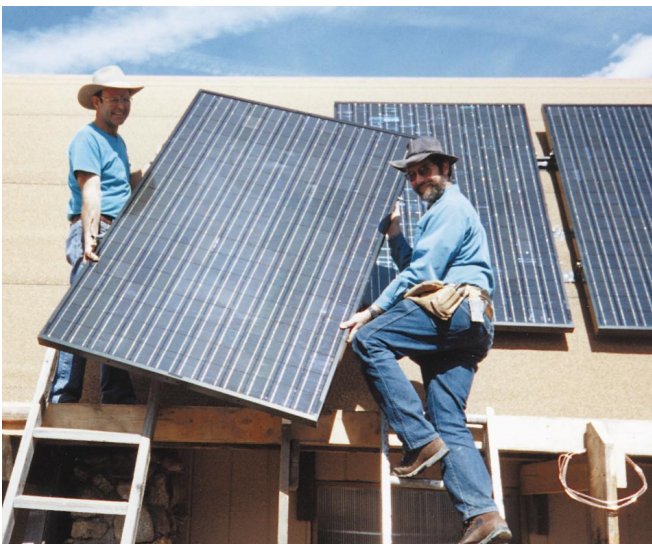
Above: Robert Warren and Don Waggoner heft a 4 by 6 foot, 245 Watt panel into place.
