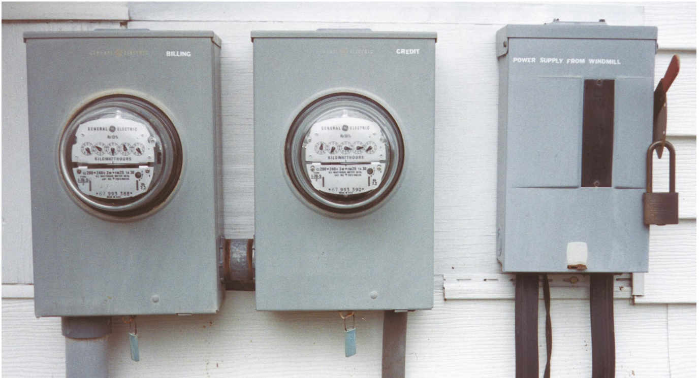
Above: The billing meter, credit meter, and lockable shutoff are located outside the house.
