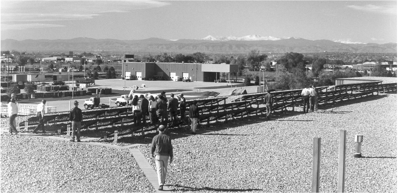
Above: The roof mounted ninety panel, 18 kW array.
