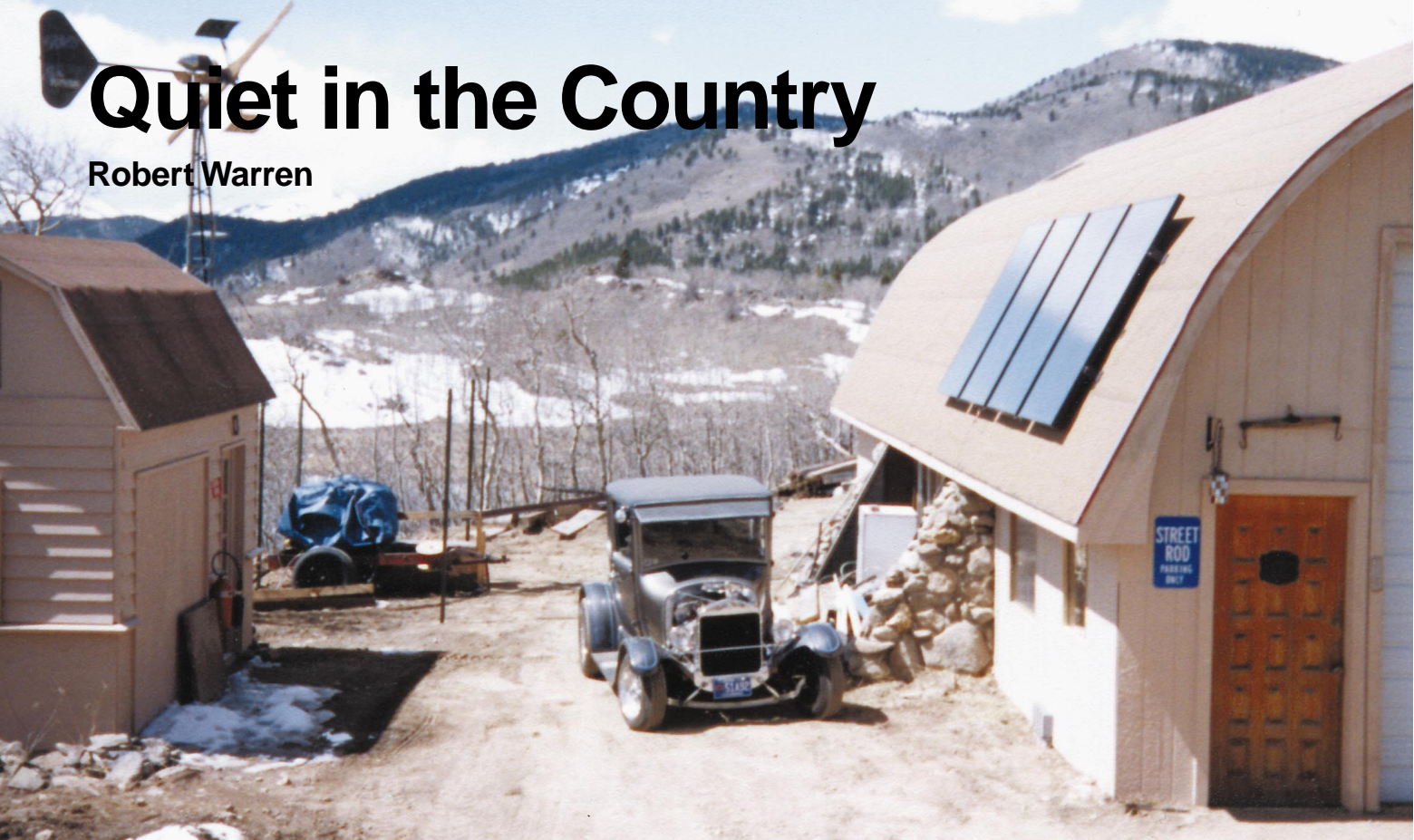
Above: 980 Watts of PV on the barn roof (right) feed the battery shed (left).
