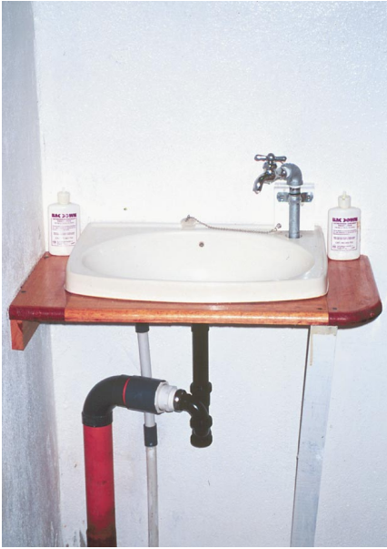
Above: Clinic sink. Faucets were also installed around the compound.
