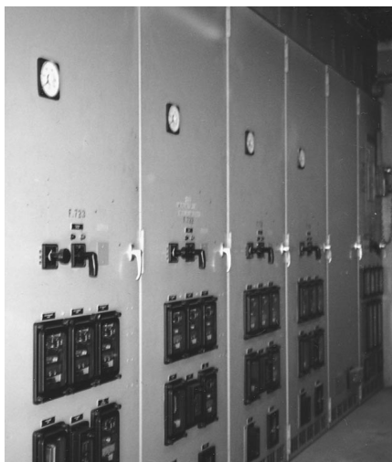
Picture 2, Left: An enclosed metal clad 13kv distribution switch gear. Each of the doors has a 3 phase circuit breaker behind it. On the door are protection relaying and an ammeter for reading each phase current.
