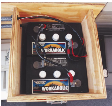
Above: A reinforced battery box holds the two 6 Volt, 350 Ah batteries.
