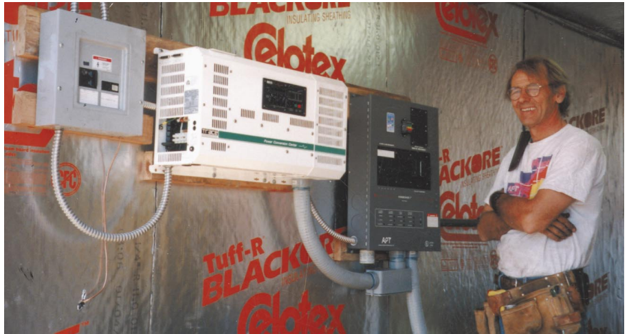
Above: Author Don Loweburg in front of the power center and inverter
