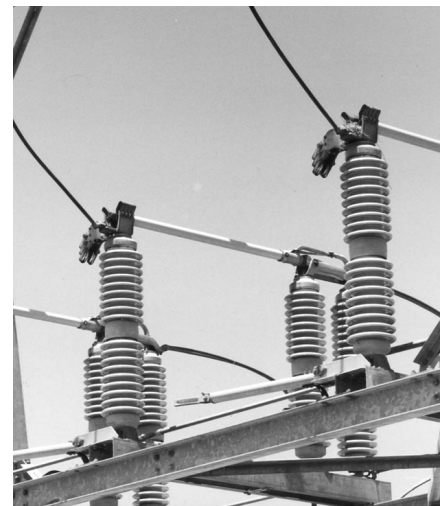
Picture 3, Right: 3 phase 138kv disconnect switches as mentioned in picture #1. These switches are in the closed position. If the switches were open (they all open together) then the horizontal long tubes between the vertical insulators would be pointed up from the back of the switch (where the wires go down).
