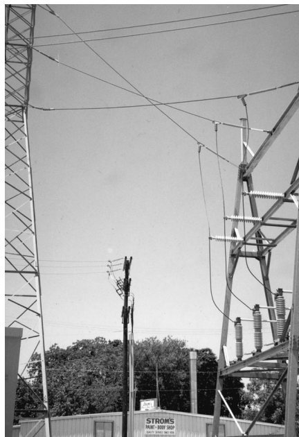
Picture 1, Above: On the left a 138 kv highline tower with conductors going to the right to a substation "A" frame dead-end. On the dead end are 138kv disconnect switches in the closed position. In the middle of the picture is a wood pole with an underground riser 3 phase pothead (that's what they call them) going through switches and attaching to a 3 phase 13kv distribution circuit. These circuits would come from a feeder breaker in the switch gear.
