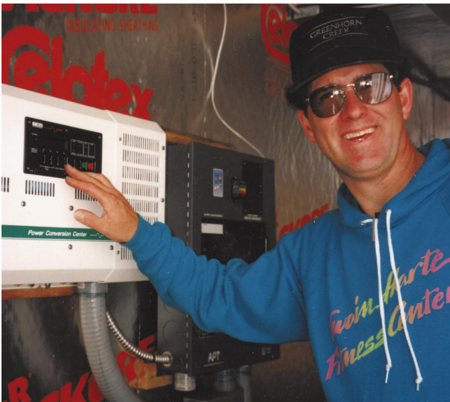
Above: Owner Don Leutz checks the power systems status on the Trace 4048's control panel.
