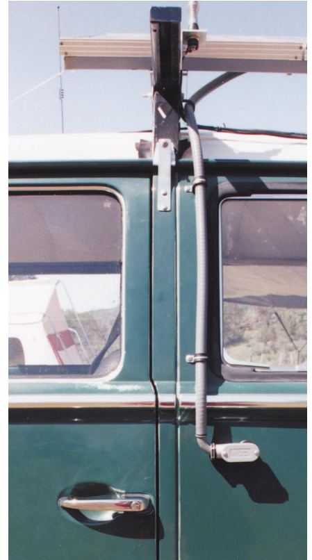
Above: A close-up view of the non-metallic flexible conduit and the bulkhead fitting into the bus.
