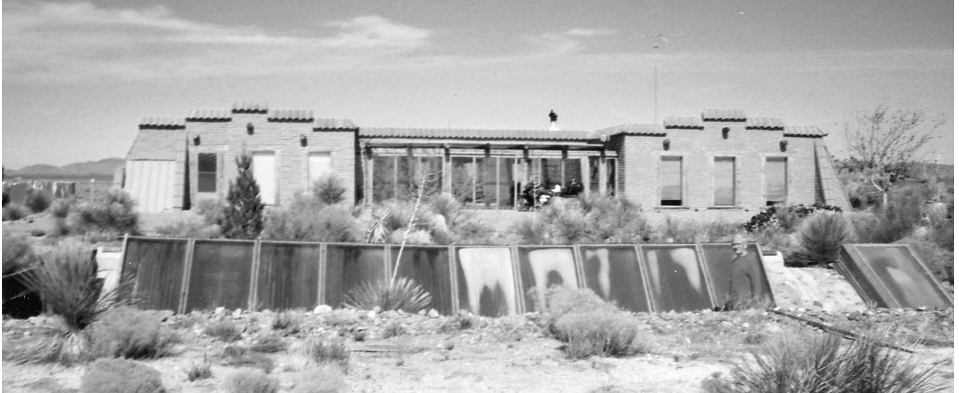
Above: Adobe house in desert setting, with ten house heating panels set into a ditch. Eleventh panel, at right, is for domestic hot water heating.
