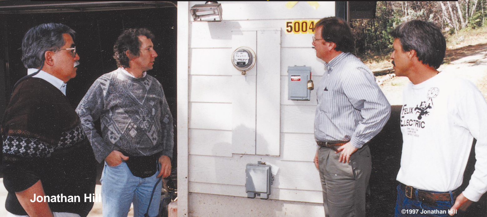
Above: From left to right, Dennis Trinidad (PG&E District Manager), Jon Hill (system owner), Clay Schmidt (PG&E account representative), and Dan Felix (electrician).
