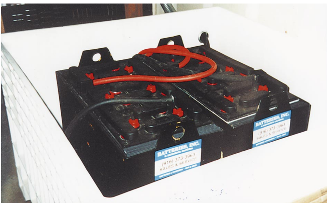
Above: Energy storage: Two Pacific Chloride 6-85-21 lead-acid batteries supplying 1055 Ampere-hours at 24 Volts DC.
