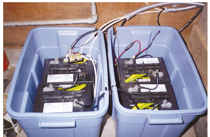
Below: Exide T-105s in spill-proof tubs.
