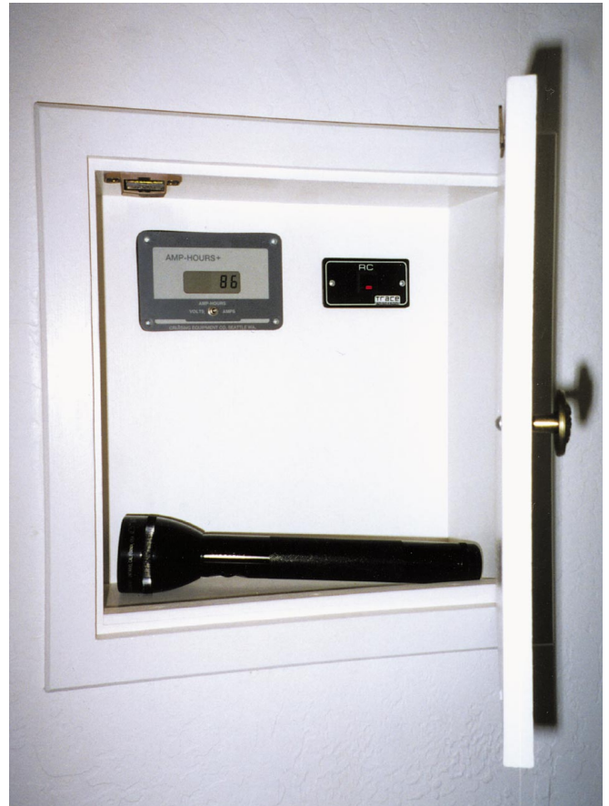
Above: The metering niche makes a handy home for a flashlight.
