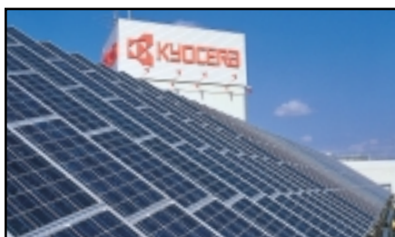
Rooftop Photovoltaic Solar System
