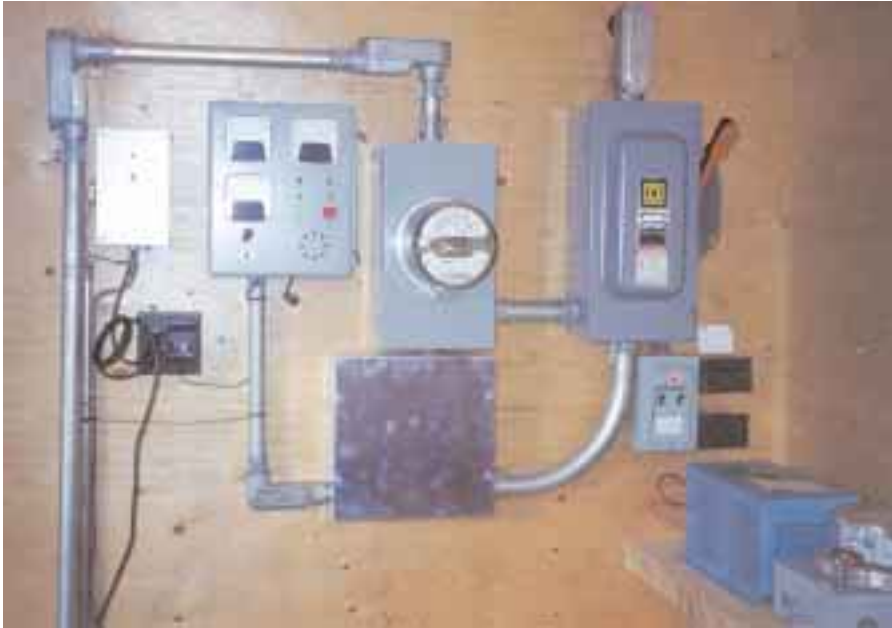
The controls and metering on the powerhouse wall.
