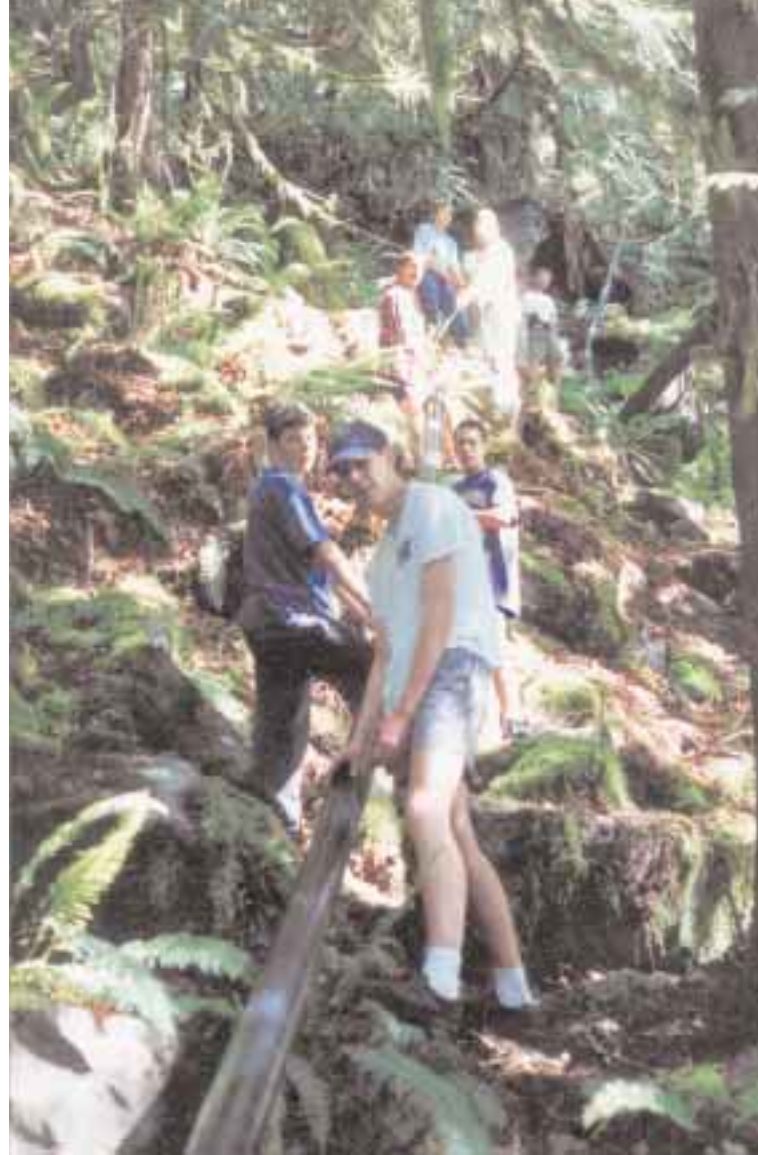
A crew of up to 25 volunteers haul 400 foot sections of polypropylene pipe up 550 vertical feet to the intake.
