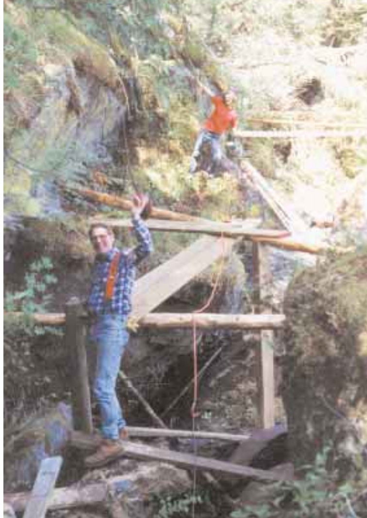
Volunteers Dave Wheeler and John Smoczyk build scaffolding to support the 180 lb. sections of steel pipe.
