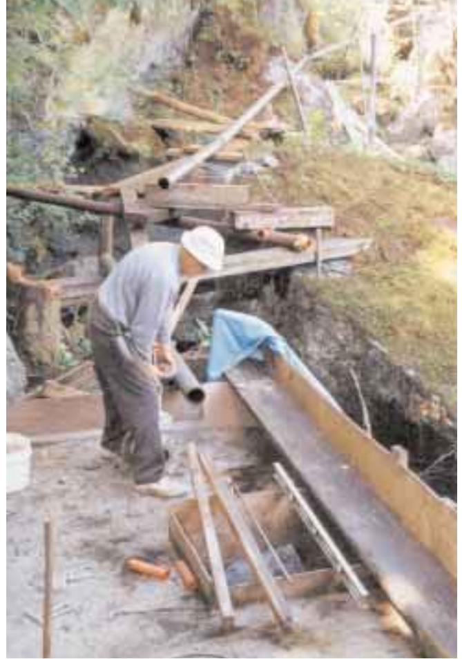
Camp caretaker Frank Poirier, on the powerhouse concrete foundation, with framing for the tailrace visible. The building was built around the turbine and generator.
