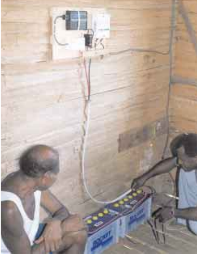
Installing batteries and inverter. Ventilation won't be a problem because there is no glass in the windows, and there are gaps in the floor to keep people cool.
