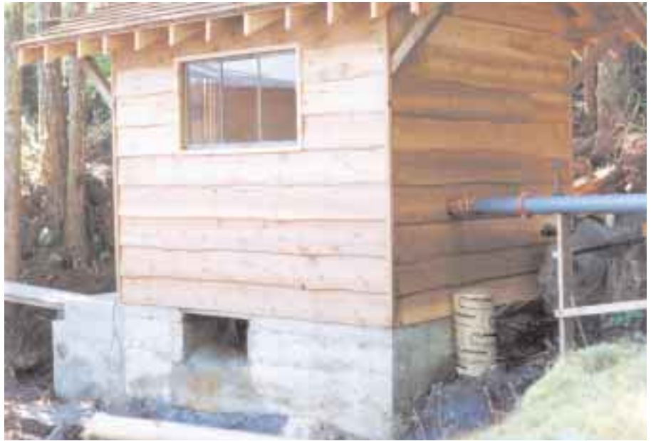
The powerhouse blends in with the forest and the traditional buildings on site. The penstock enters the rear of the building.
