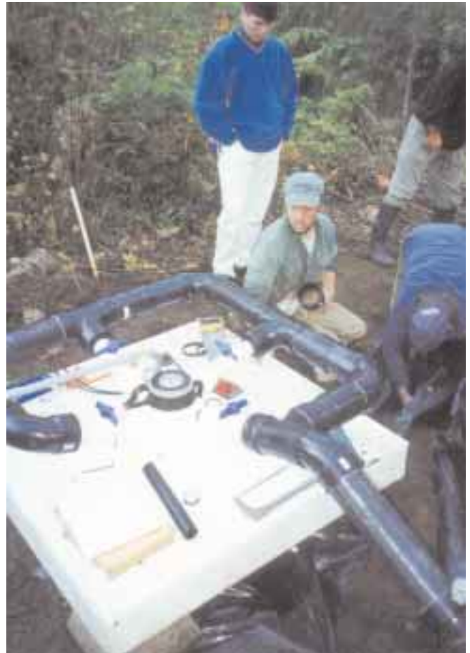
The completed manifold with the ES&D turbine.
