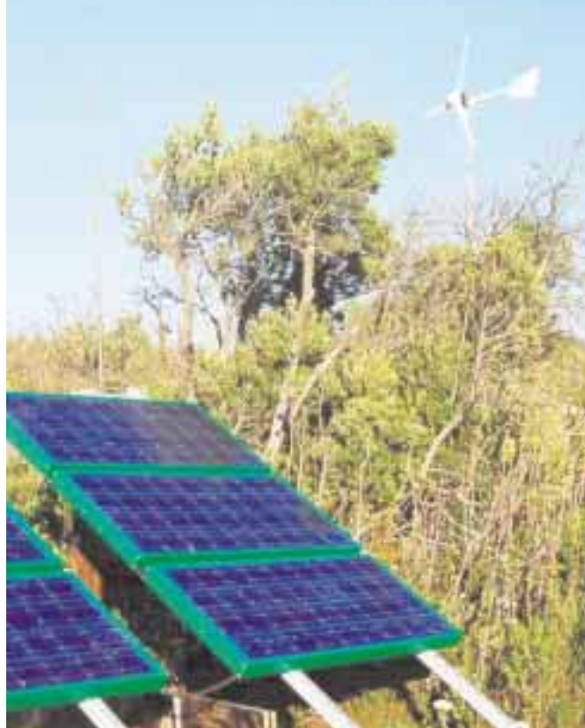
The African Windpower bird above the telecomms array.
