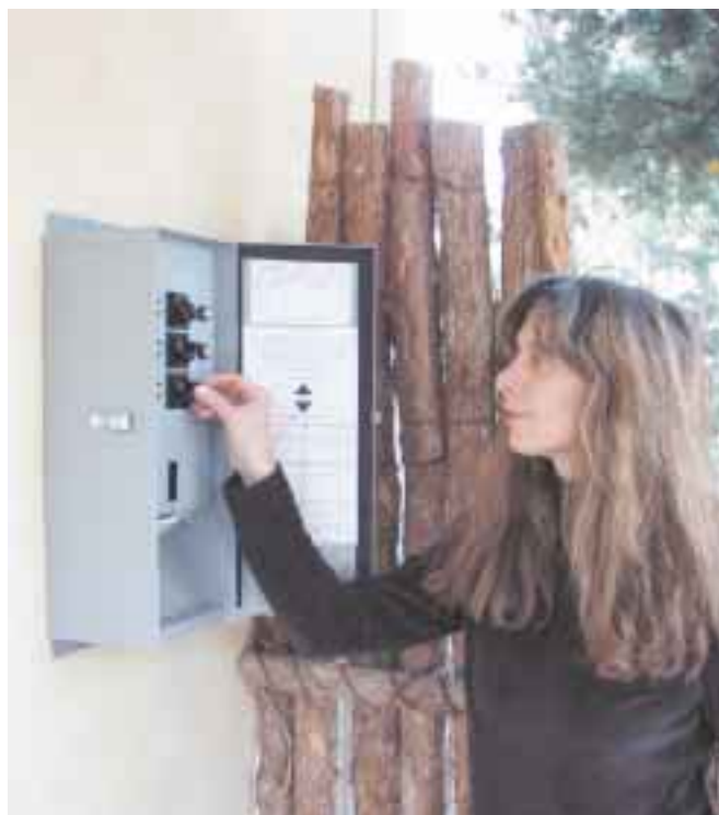
Anne flips a switch in the transfer box—part of the house is now running on solar power. The label identifies the loads carried by each switch.
