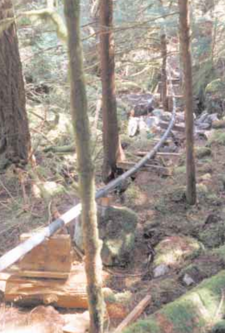
Down through the trees, the bottom sections of steel pipe reach for the powerhouse.
