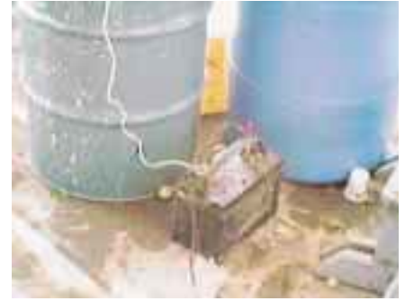
A solar-charged 12 volt battery powers the mixing process.
