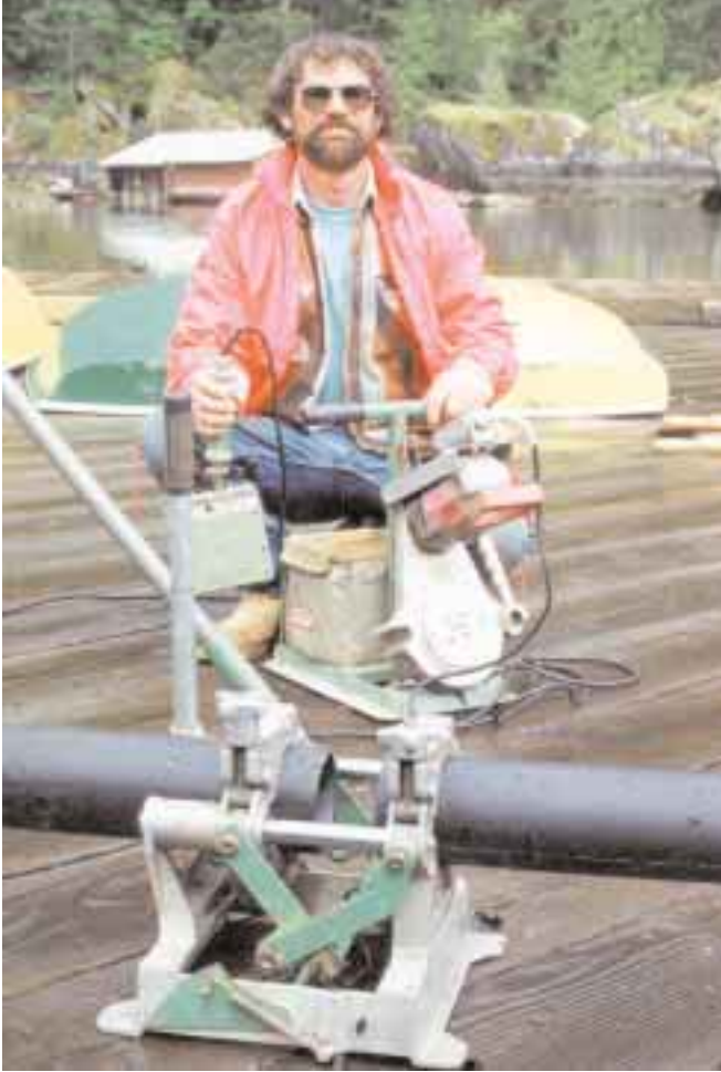
John Smoczyk, a regular volunteer at Malibu, shows off the fusion welding equipment for the polyethylene pipe.
