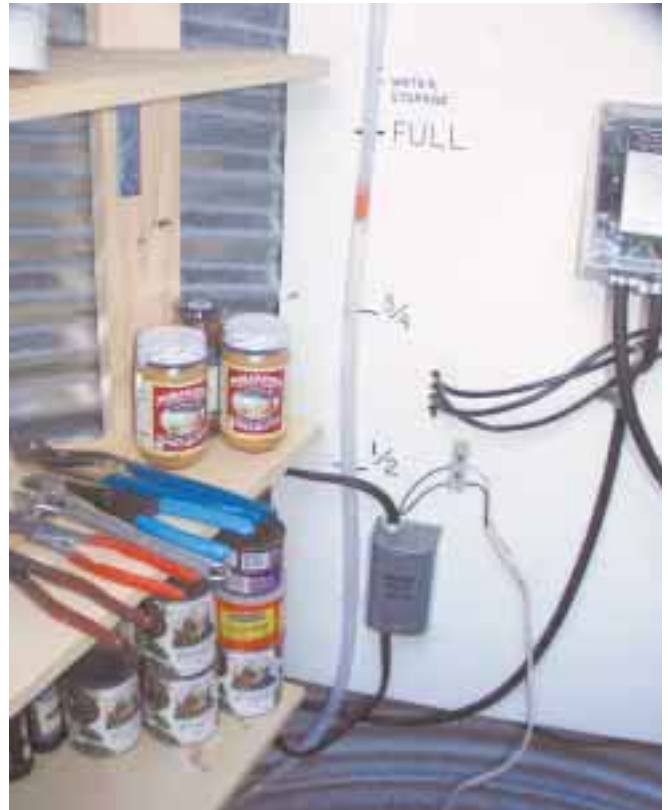
Inside the well pit is this sight tube. The orange float indicates the level of water in the storage tank. The well pit is also used for food storage.
