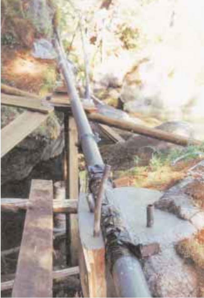
The thrust block at the powerhouse keeps the tremendous weight of pipe and water from sliding downhill and crashing through the building.
