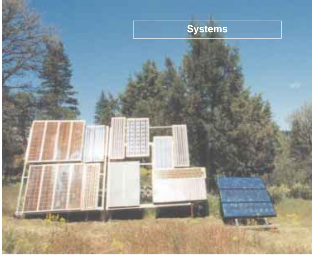
12 volt PV sub-array #2: The democracy rack and more, 580 rated watts.
