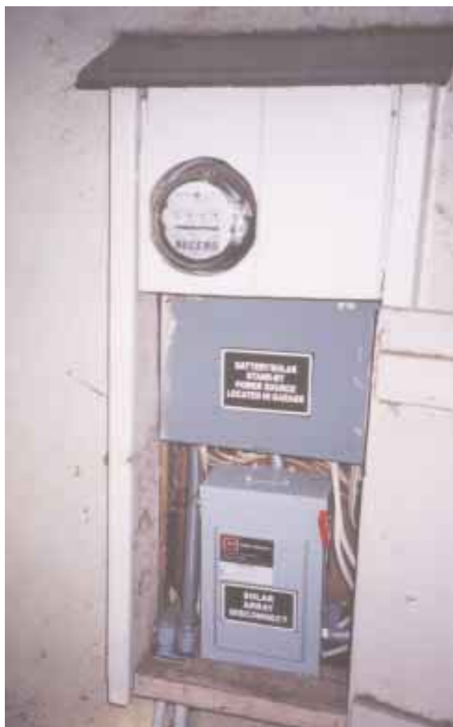
Outside—the utility KWH meter and lockout.
