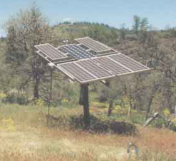
12 volt PV sub-array #3: 310 rated watts.
