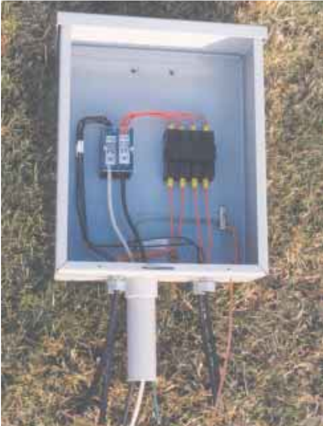
Combiner box with midget fuses, fuse blocks, and safety pullers.
