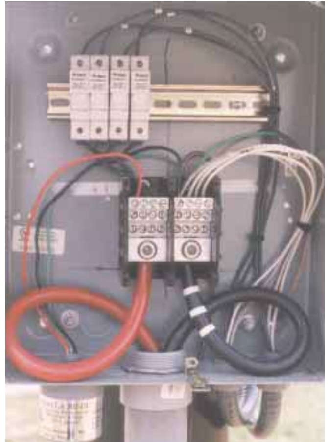
A combiner box for an array with four series strings, designed and constructed by Shawn Fitzpatrick.
