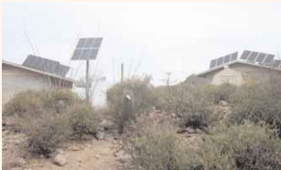
Photovoltaic systems at the Cooper Environmental Sciences Campus, where the classroom part of the workshop took place.
