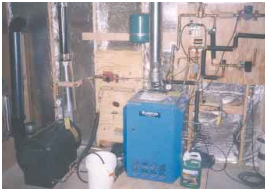
A Buderus boiler (right) provides hot water for space heating. A Hot Products wood-fired boiler (left) preheats the water.
