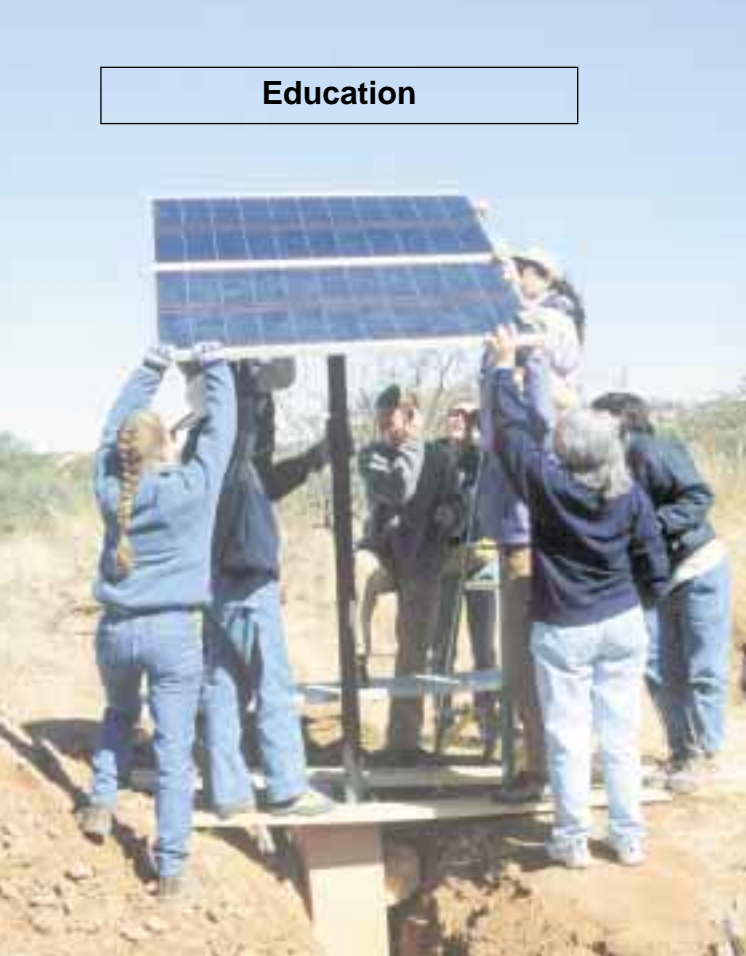
Students mount the two Uni-Solar 64 watt PV panels at Darlene's remote desert home.
