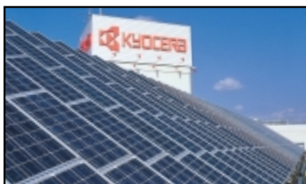
Rooftop Photovoltaic Solar System
