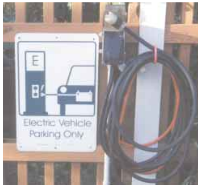
Will's EV charging station.
