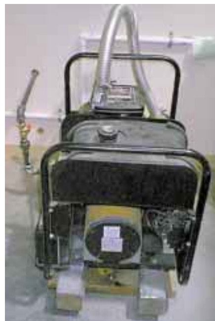
The Winco 9,000 watt backup generator runs on propane.
