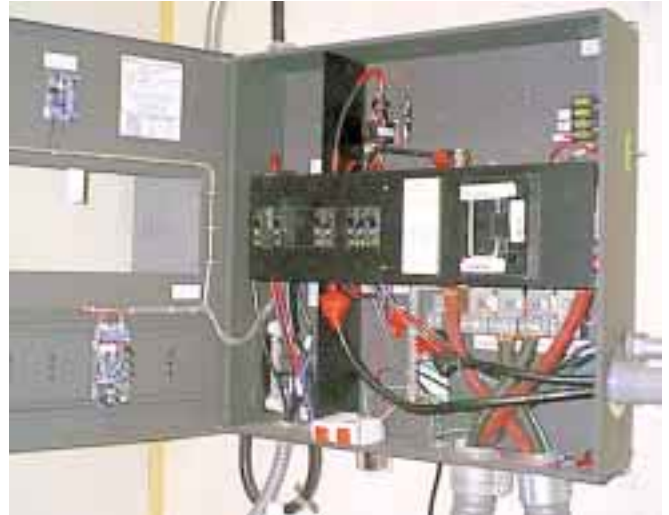
Inside the Ananda Power Center you can see the main pullout DC disconnect, DC breakers, and the backs of the TriMetric and Smart Charger.
