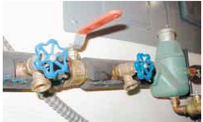
Three valves make up the drain/fill assembly.
