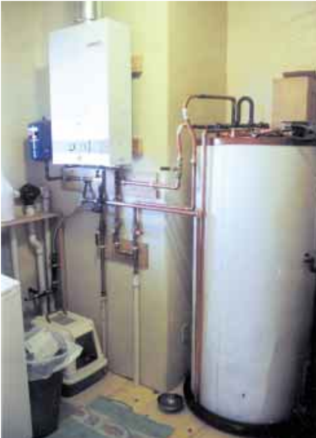
An Aquastar BS on-demand water heater (upper left) backs up the solar hot water system.
