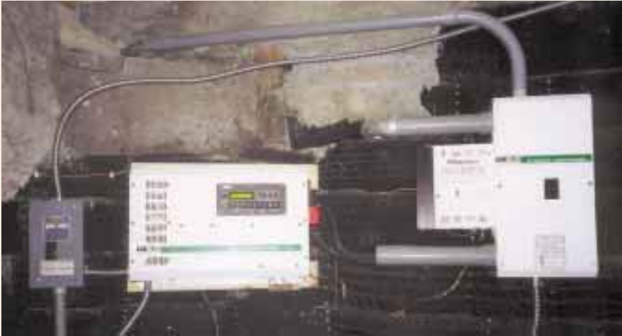
The Trace SW4024, RV Power Products SB50, and Trace DC250.
