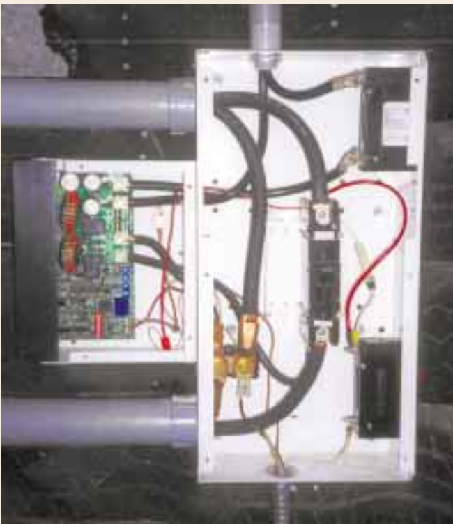
Inside the SB50 and DC250.
