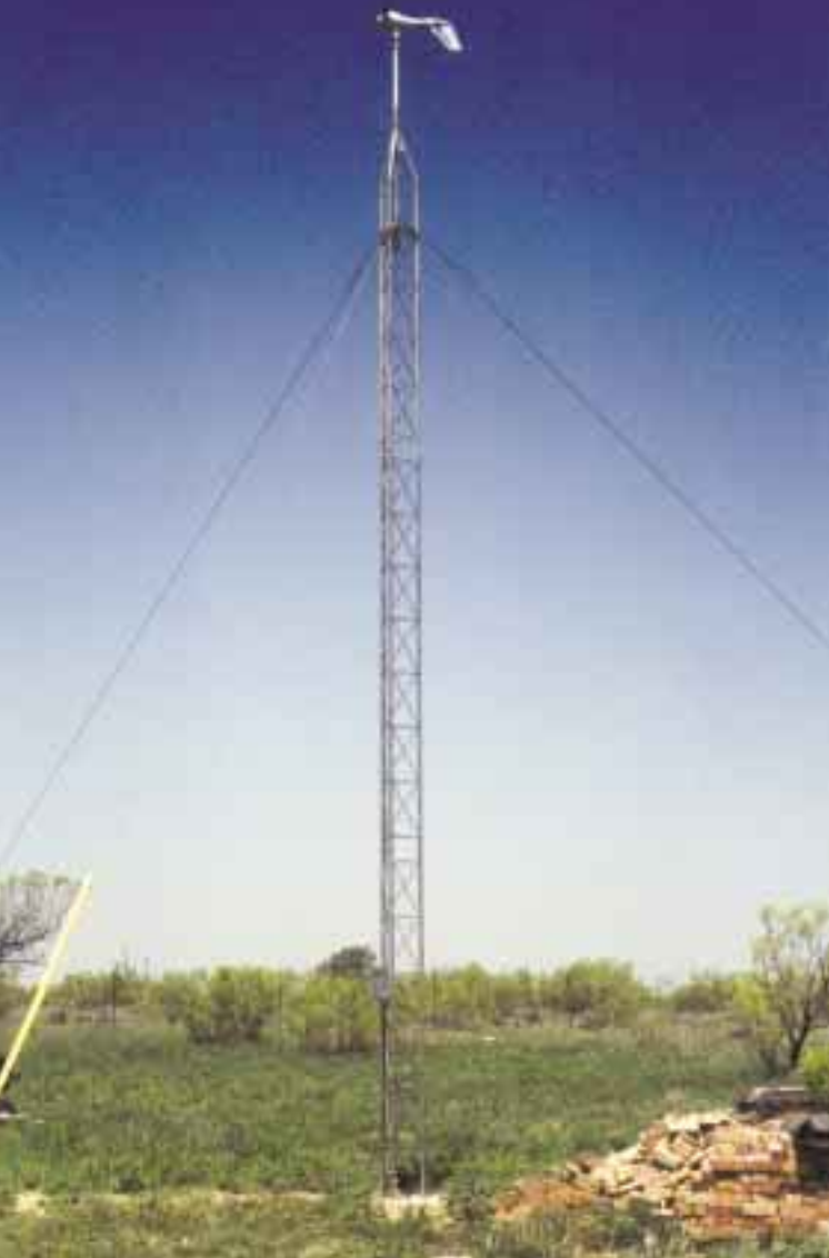
The Southwest Windpower Air 403 on a 30 foot tall Rohn 25G tower.
