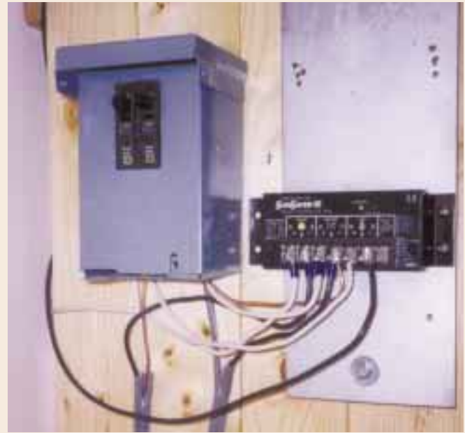
Breakers and the Morningstar SunSaver-10 charge controller for the 12 volt system.
