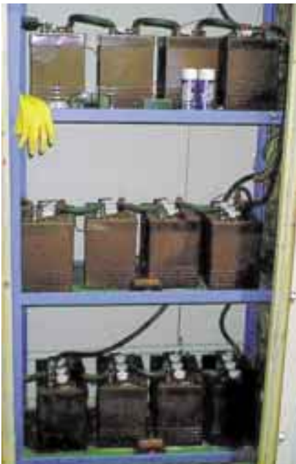
Twelve of the sixteen Trojan T-105 lead-acid batteries that provide 880 amp-hours of storage.
