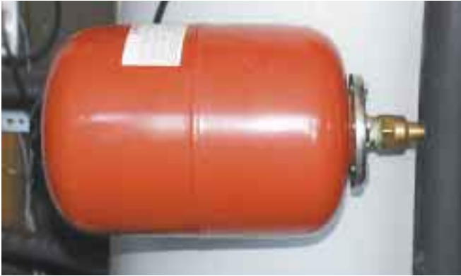
An expansion tank maintains pressure in the closed loop as system temperature changes.
