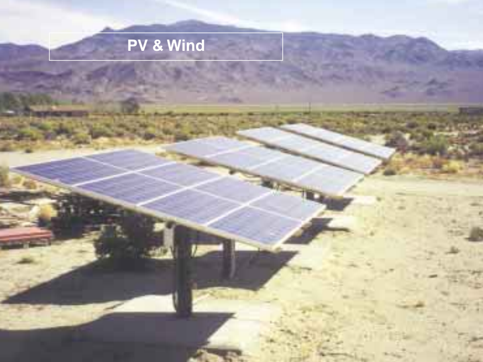
Thirty-two of the ninety-six PV panels are on stationary mounts.
