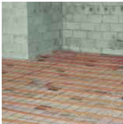
Basement during construction, showing 2 inches (5 cm) of insulation on the floor and radiant floor tubing. The repaired holes in the cement block are where expanding foam insulation was injected inside the 12 inch (30 cm) blocks.
