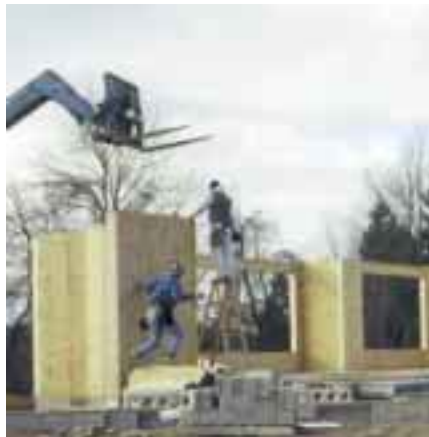
Structural insulated panels (SIPs) form the entire house structure. A small crane sets the SIPs into place.
