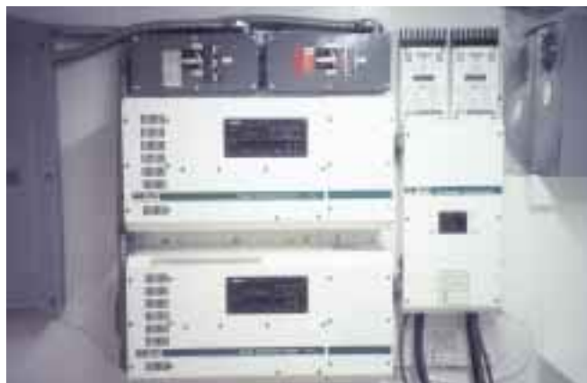
Power panel #2 for 32 PV panels and the wind generator.
