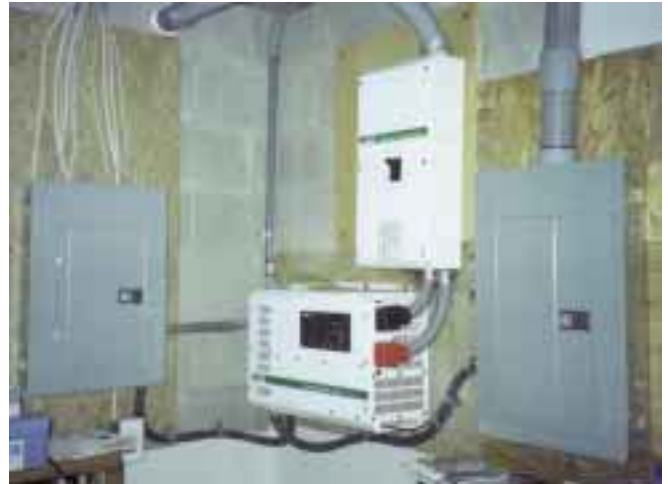
The DC disconnect box, inverter, and two subpanels are located in the basement, and the batteries are in the garage above.
