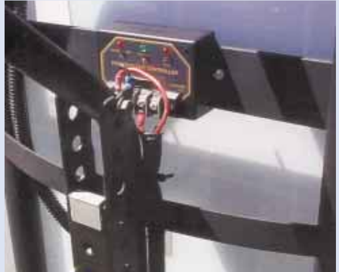
A close-up of the PV charge controller.
