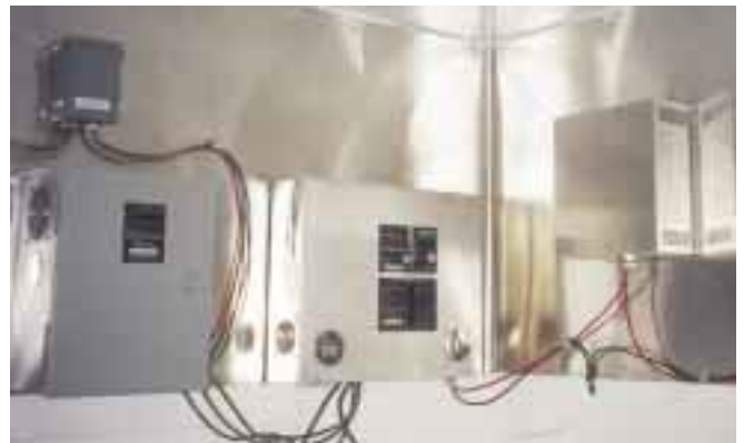
The Whisper EZ-Wire Center, step-down transformer, and diversion load heater box in the power room.
