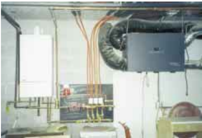
The natural-gas-fired boiler (left) and heat recovery unit (right). Note the basement ceiling is Spancrete.
