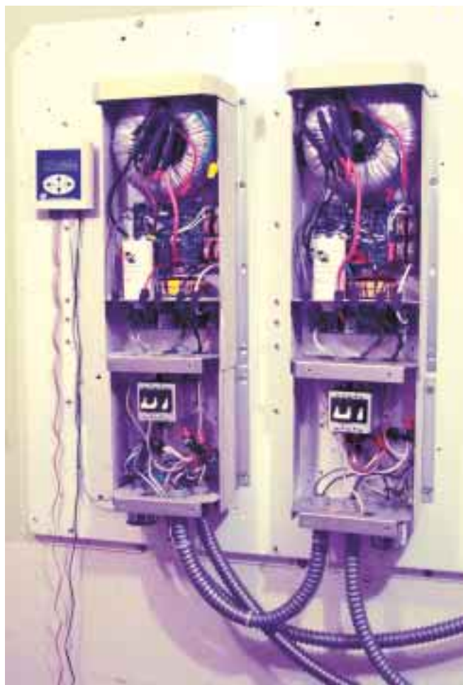
Advanced Energy's AM100 Inverter Monitor (left) and the interior of the GC-1000 inverters.
