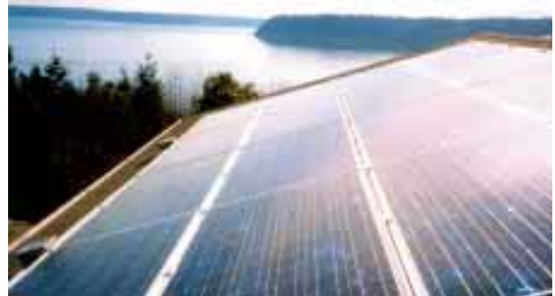
5 KILOWATT GRID-TIED PV SYSTEM
