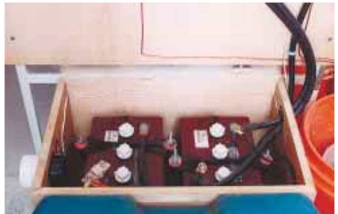
The system's two lead-acid batteries are vented and safely secured for travel.
