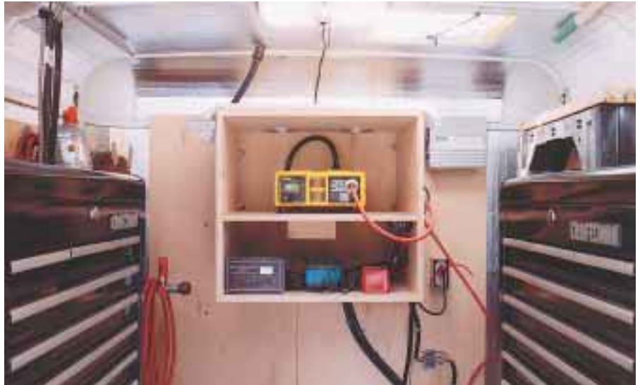
The RE equipment: inverter (center, top shelf), AC battery charger (upper right), and PV charge controller (left, bottom shelf).
