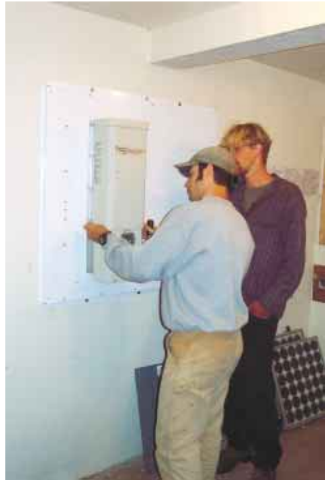
Andrew Posner and a student installing the first Advanced Energy GC-1000 inverter.
