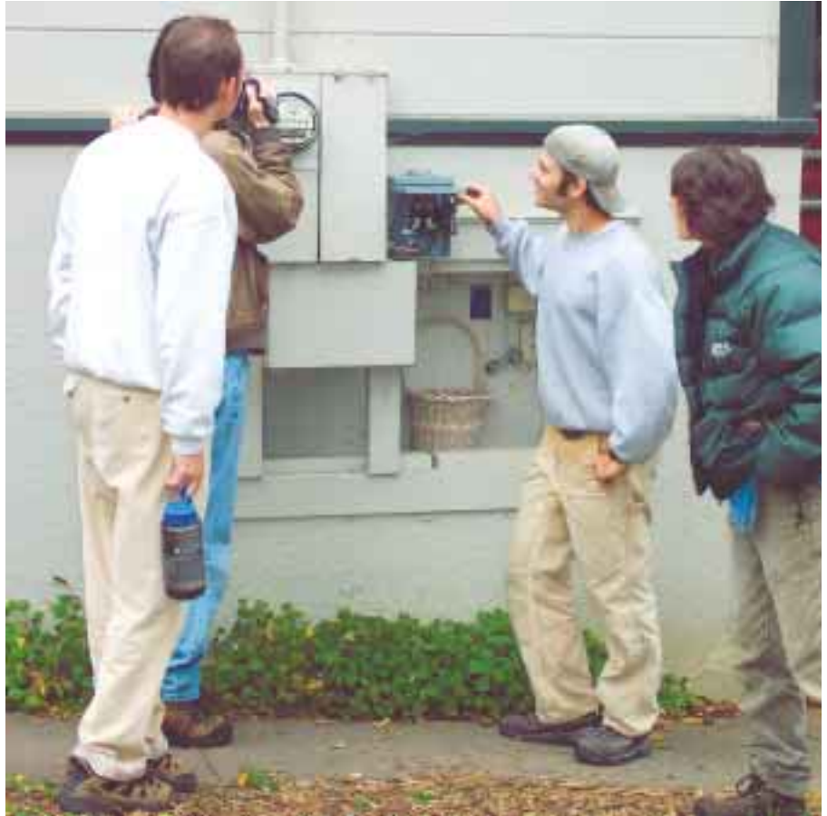
The crew testing the utility's lockable disconnect switch—and watching the utility meter spinning backwards!
