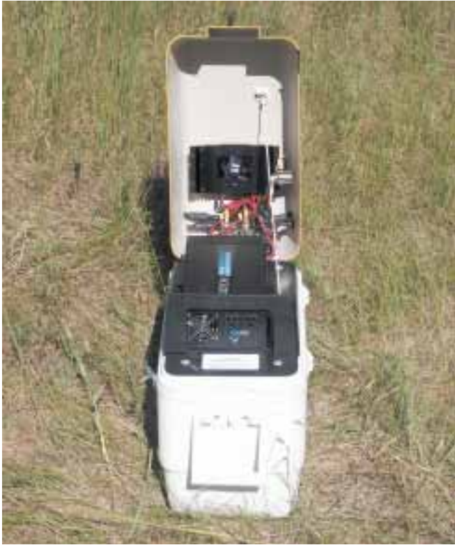
A 600 watt Exeltech inverter provides high quality power. The AGM battery is housed below in an insulated space.
