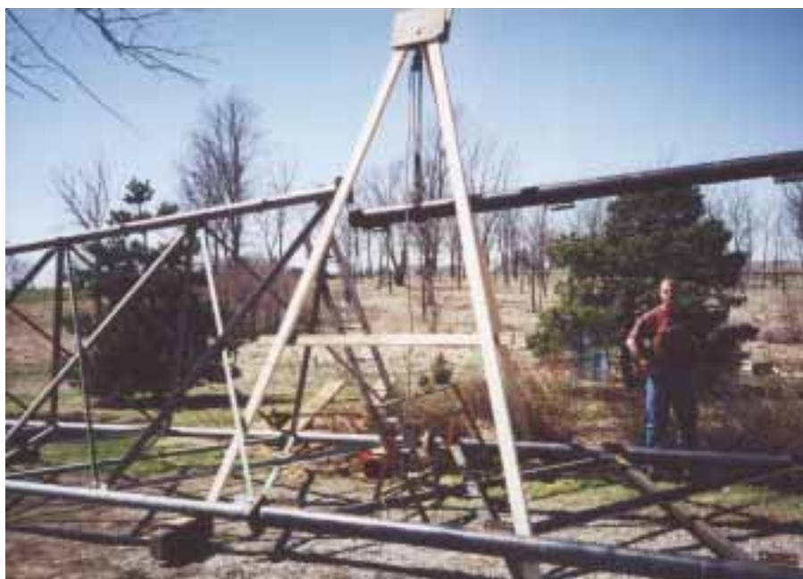
The 40 foot sections were assembled horizontally. Tripods, a winch, and block and tackle were used to position the 300 pound legs for welding.
