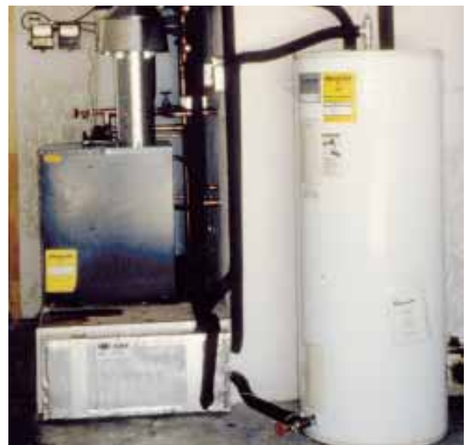
A shell-and-tube, double-wall exchanger in an insulated box on the floor.
