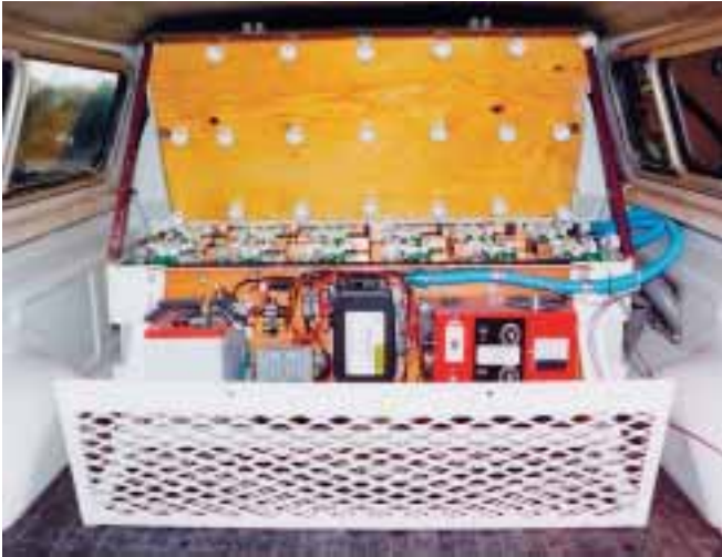
In the pickup's bed, Joe and Emily designed a custom space to safely carry the batteries and components that wouldn't fit under the hood.
