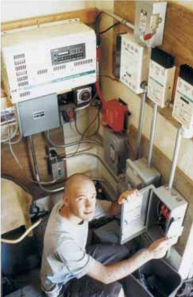
The control room—Trace SW4024, two Trace C40s, RV Power Products SB50, E-Meter, disconnects, and overcurrent protection.
