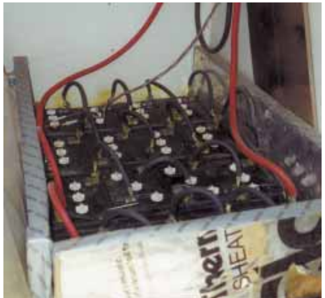
Sixteen Trojan L-16s store 1,400 AH at 24 V. The batteries are in a separate room, and are well insulated (a removable blanket of fiberglass insulation is added during the winter months).
