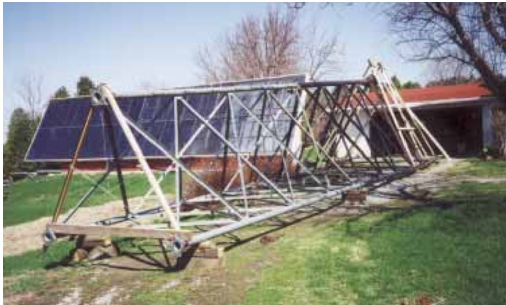
Don's homemade, 20 foot bottom section (black, background) is attached to the original Rohn, 20 foot bottom section (silver, foreground).
