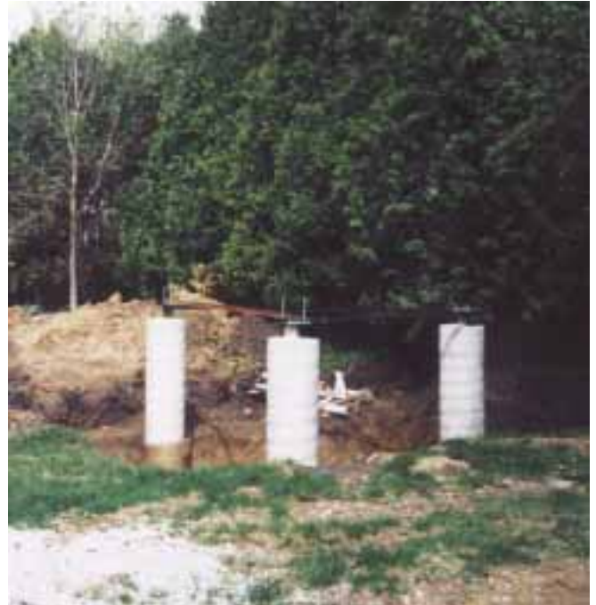
Three concrete and rebar piers, poured around 8 foot angle iron legs, are embedded in the foundation.
