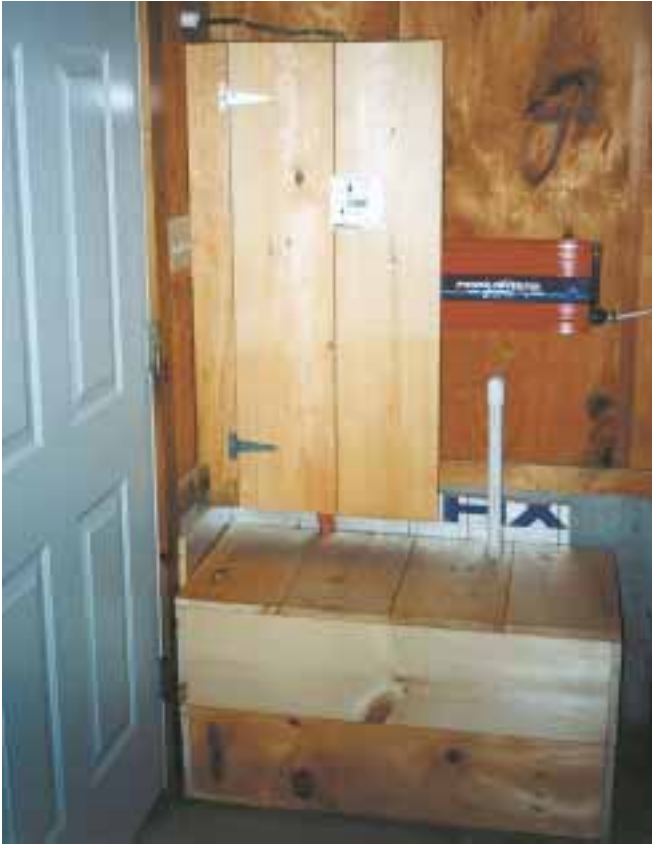
The battery box is safely vented and enclosed below the power center.
