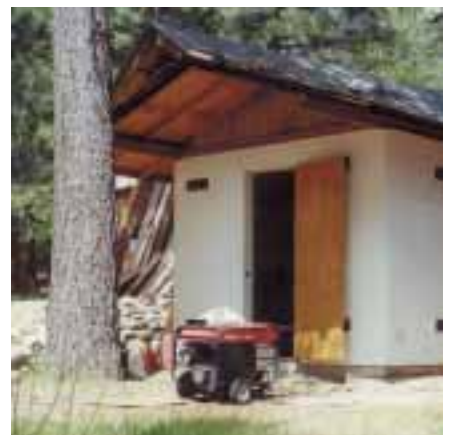
A power shed in the pines with the Honda ES6500 engine generator outside. The Honda acts as a second backup.
