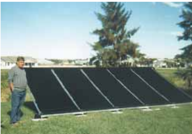
Solar pool panels—ground mounted.
