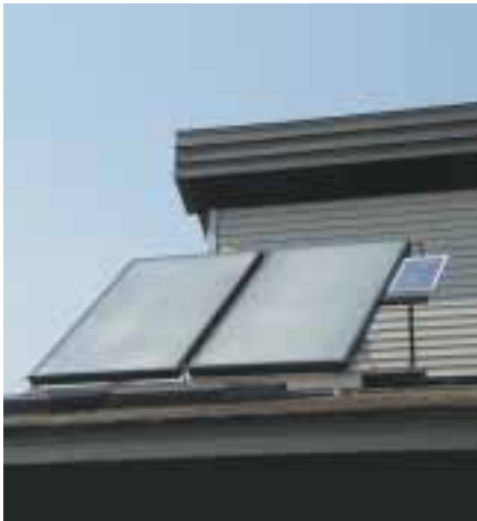
Rack-mounted, PV powered system.
