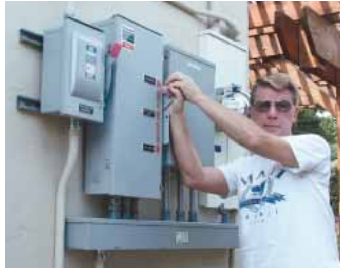
Brent Simons throwing the switch at the AC service panel.
