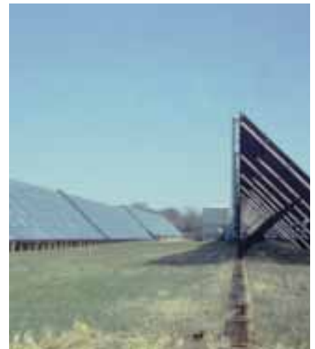
Ground-mounted commercial system.
