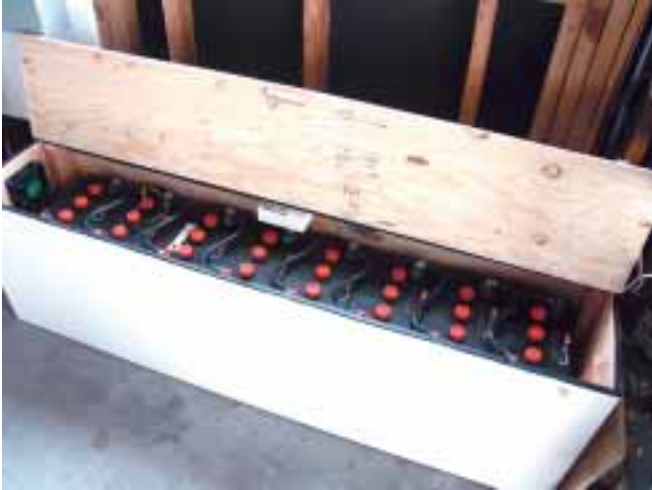
The battery bank provides ample backup to critical loads.
