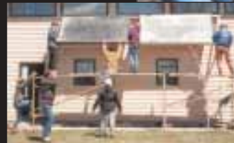
Solar Hot Water
