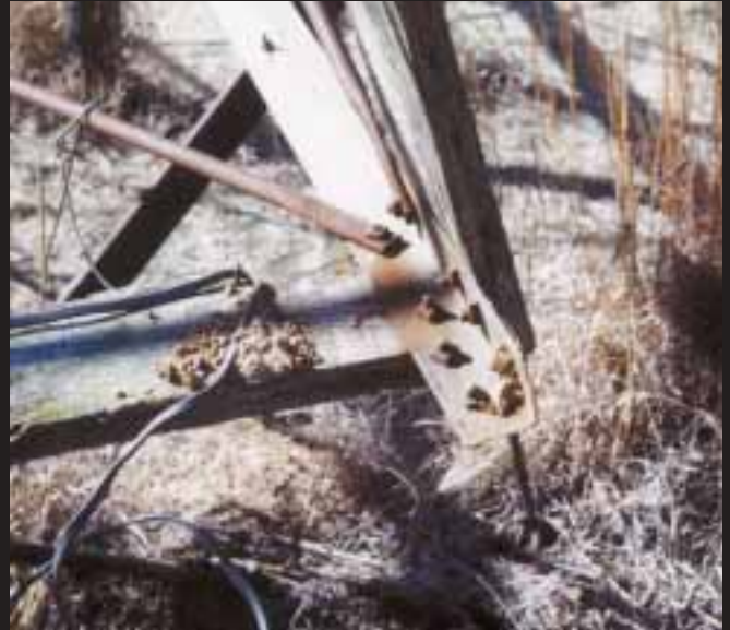
All four tower legs looked like this—completely and squarely rusted off, right at ground level.
