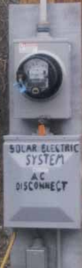
The utility meter and lockable disconnect are the only stationary parts of the system.
