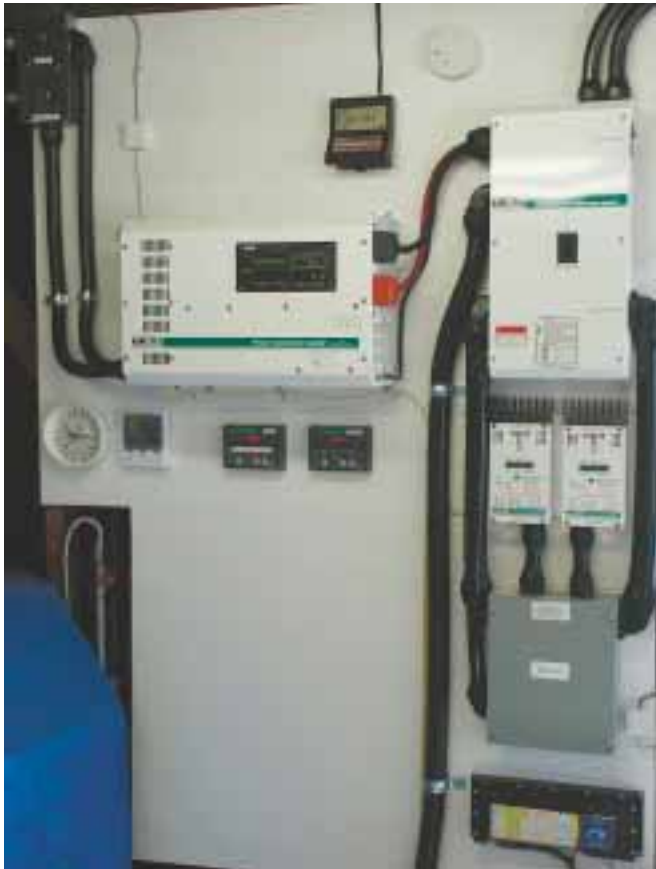
The power panel is installed in the garage.
