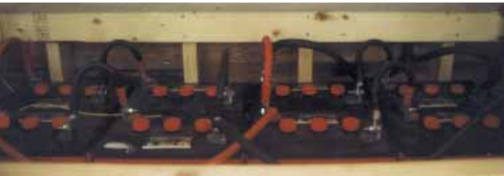
Eight, Surrrette S-460, lead-acid batteries provide ample energy storage.
