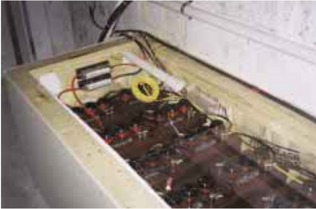
Eighteen Trojan T-105s make up this battery bank. The battery system is insulated, fused, and vented.
