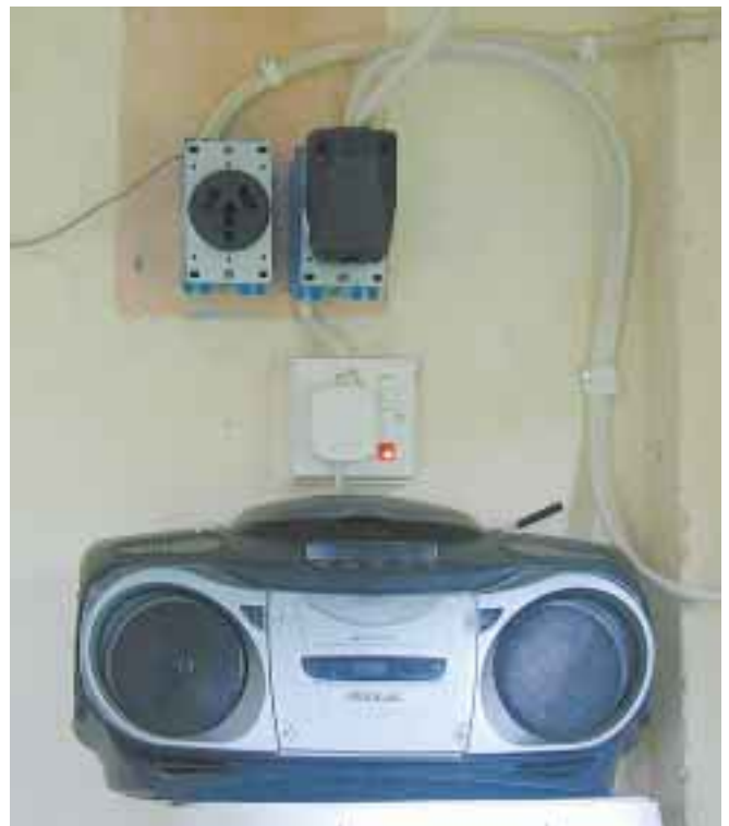
Two 230 V receptacles allow a choice between utility or generator power. The LED and stereo indicate a hot grid.
