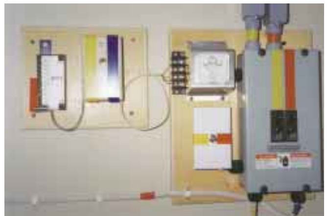
The author's first try at the house's east wing monitoring and distribution panel—before he added conduit.
