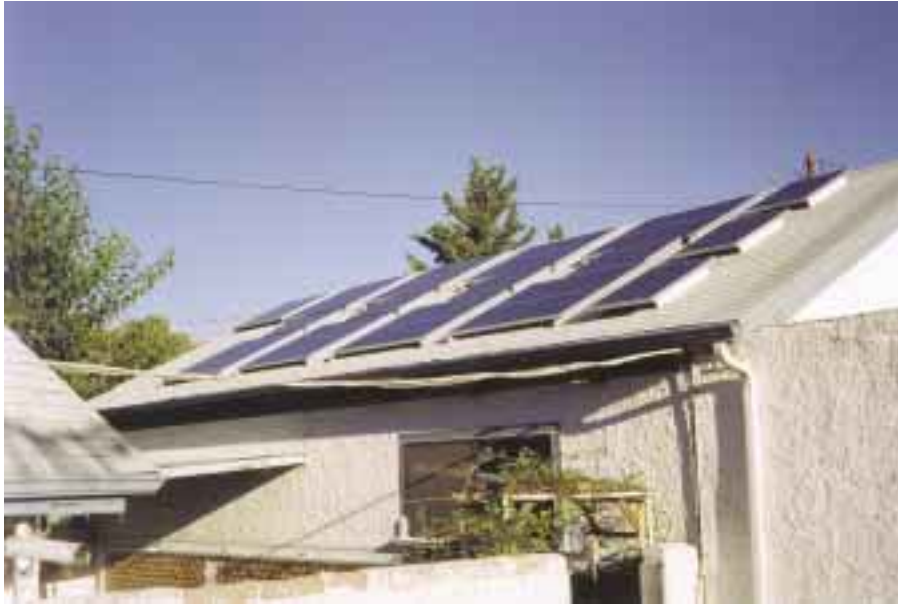
From three panels to twenty-five—the system keeps growing, and growing, and growing! The sixteen KY120, seven KY80 and two SP75 PV panels.
