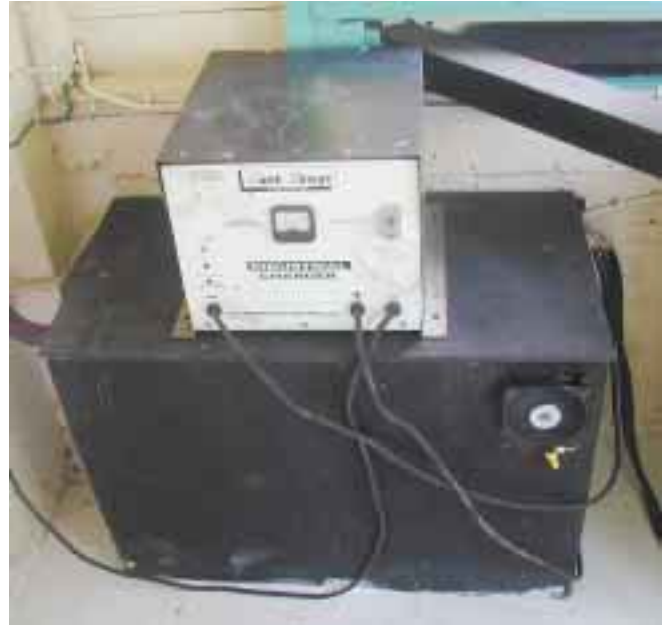
The AC charger, used for grid backup, sits atop the vented battery box that holds four Trojan L-16Hs.
