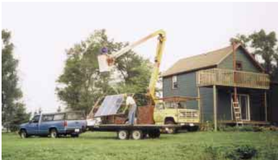
Moving the PVs wasn't too hard with the help of this cherry picker.
