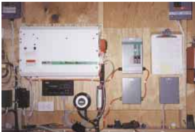
The Trace PS2512 inverter, the AC-in breakers and isolation box. A PV amp-hour log is kept on the clipboard.
