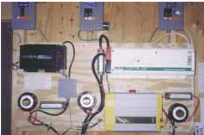
The Trojan system's inverters: XP600/12, PROsine 1,000 watt, and DR1512.
