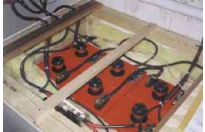
Three of the twelve Roll's batteries. The #4 (21 mm 2 ) wiring shown is from the C60 controllers.
