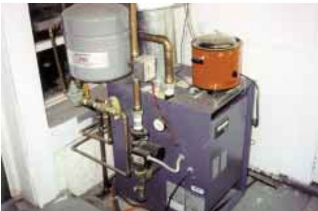
The Weil-McLain furnace with its little pump.
