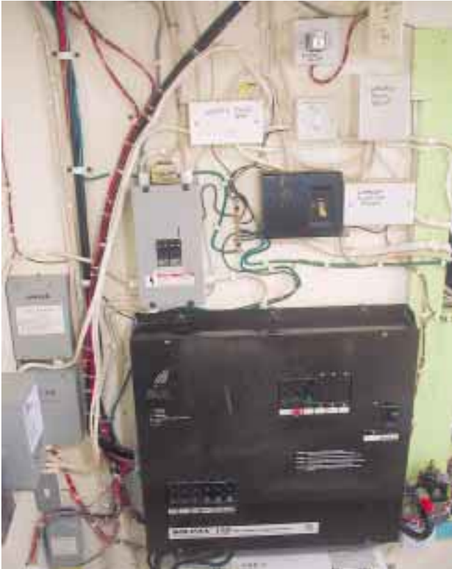
The power wall including the SolPan 110 DC load center, which contains a Heliotrope CC-120 charge controller.
