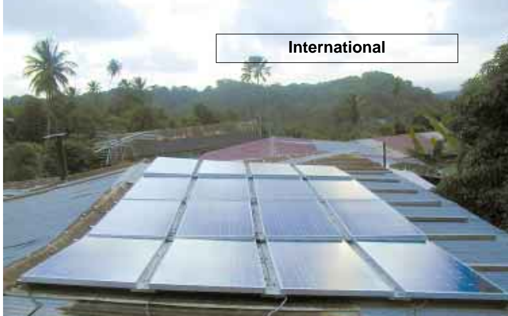
Sixteen, 120 watt AstroPower modules provide power directly to DC-driven, chocolate making machines.
