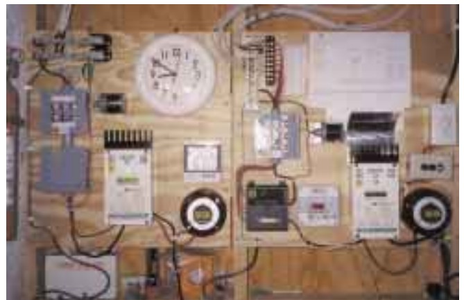
Part of the system's power wall, including Trace C40 and C60 charge controllers, instrumentation, and overcurrent protection.
