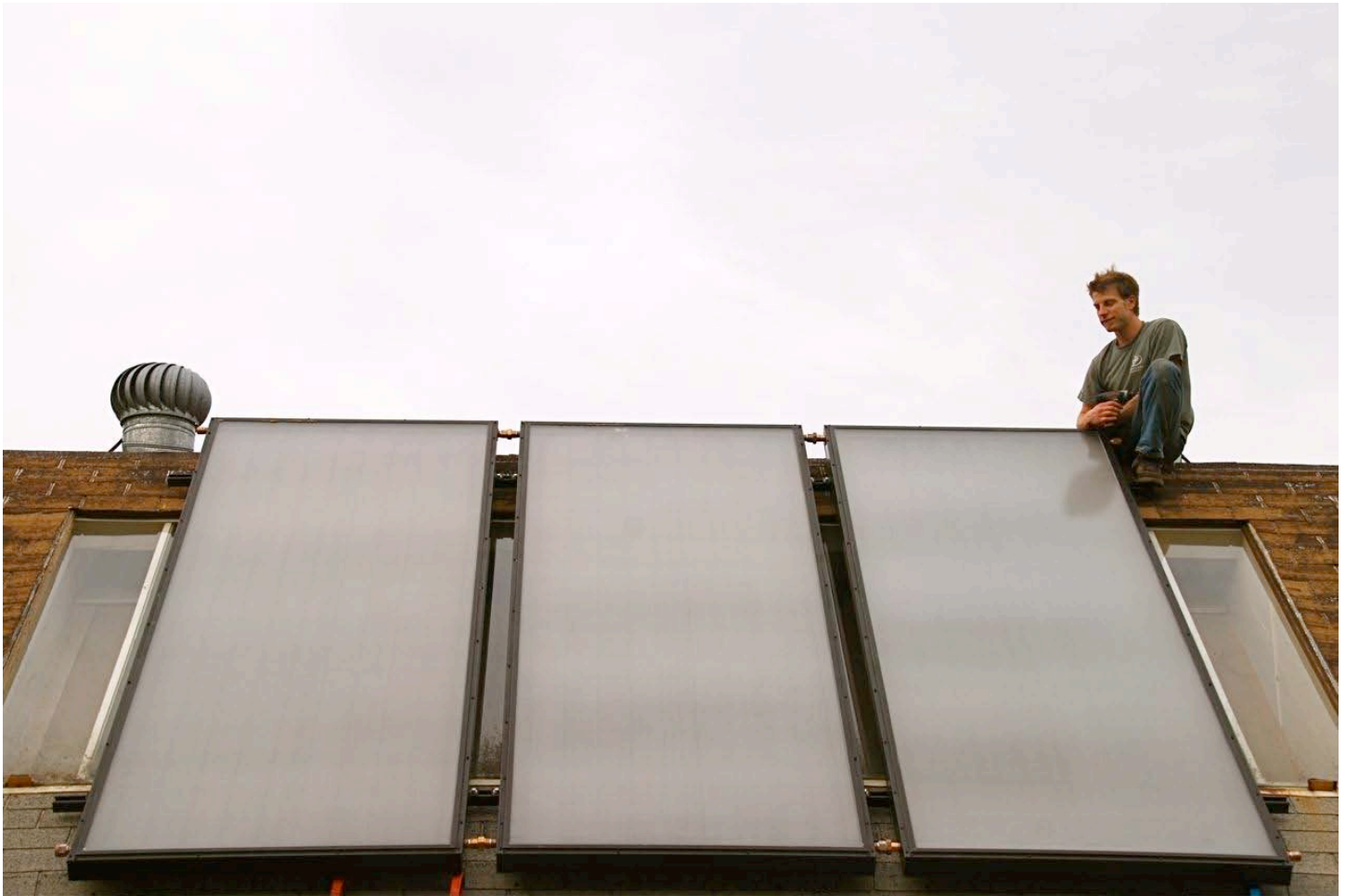
Solar hot water panels mounted on the south-facing roof of the Guest Bath House. Photo: Jim Coleman
