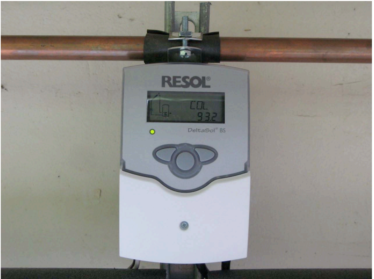
Differential temperature controller Photo: Brock Dolman
