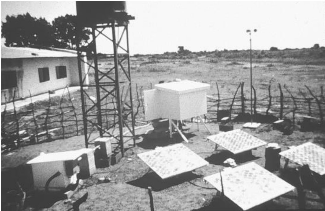
Figure 6: PV can be used to power water pumping systems ©ITDG
